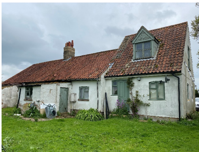
Looking to the rear of the property towards painted brick rear lean-to extensions
