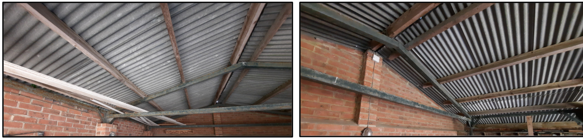
Plates 3 a to c – Internal Views showing roof covering, steel frame and purlins.
