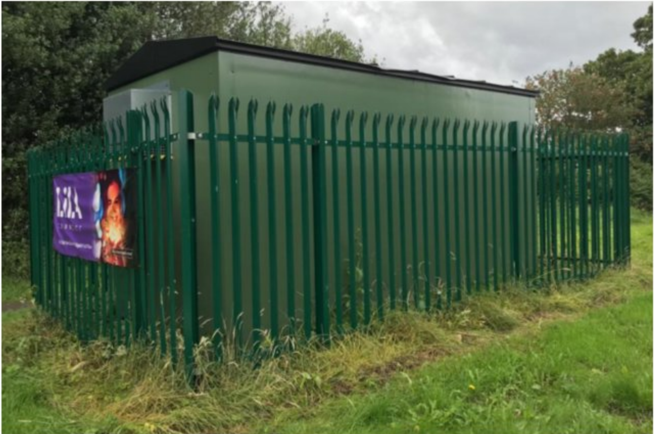
Photograph 1: Telecoms Shelter and Security Fencing in situ
