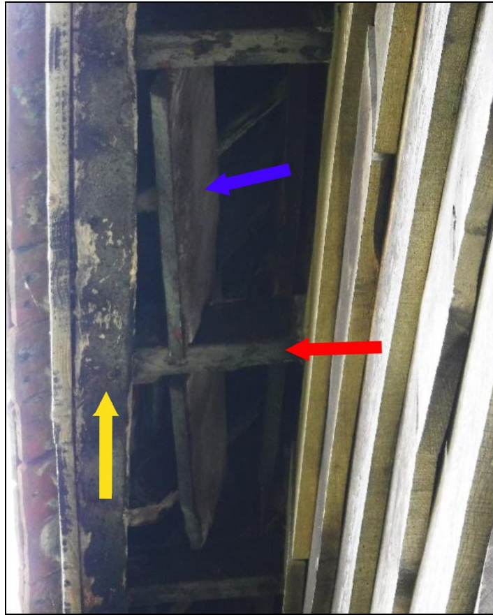
Figure 14 View up under the eaves showing the short horizontal timber struts (red arrow), the external rail (yellow arrow) and one of the near vertical boards that may be remnants of a ventilation scheme (blue arrow)
