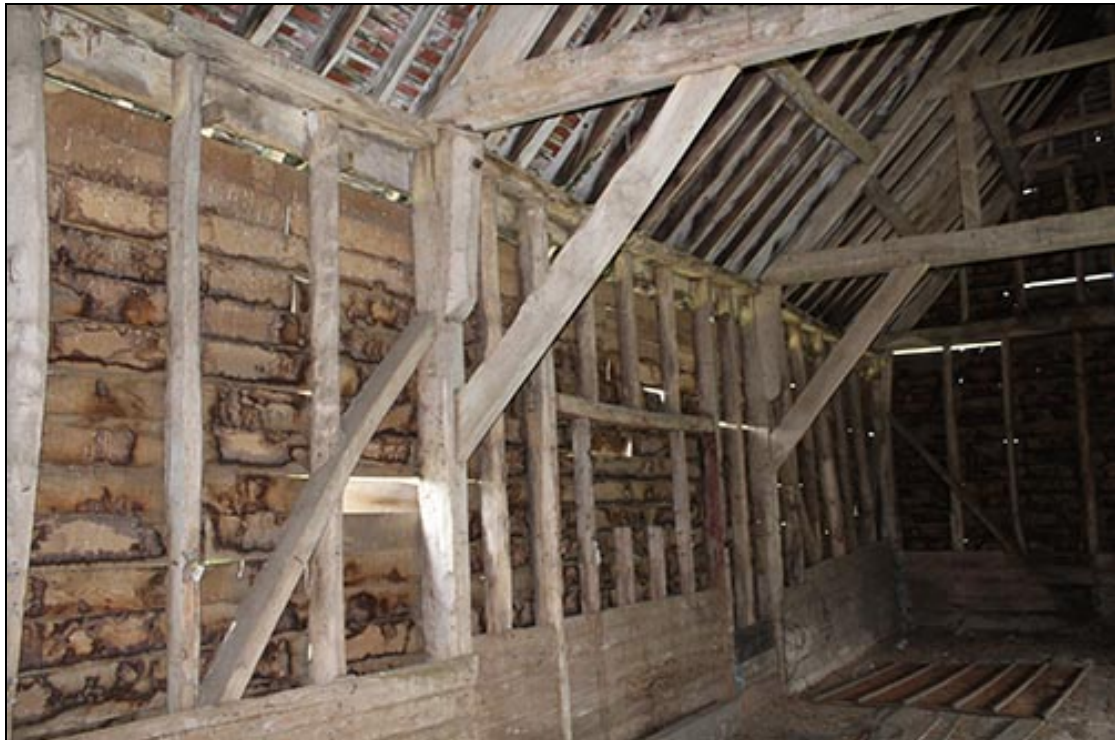
Figure 15 The south wall of the Threshing Barn looking west and showing the surviving elm boards just below the wall-plate, together with the infilled south door in the central bay
