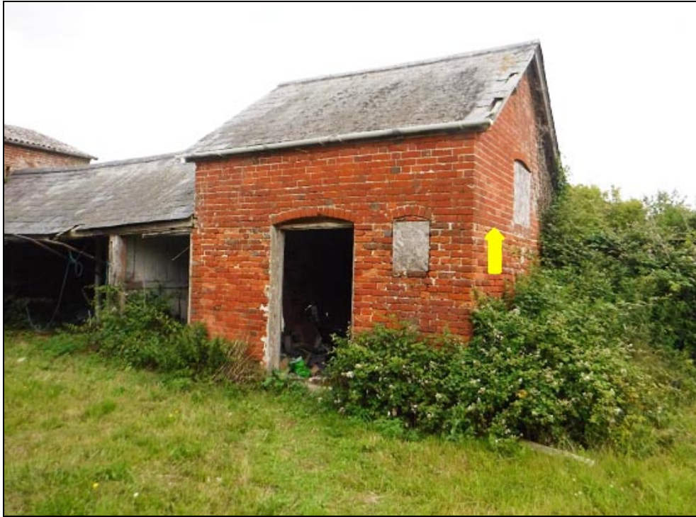
Figure 29 The Small Store looking north-west, with the height of its original brickwork indicated by the yellow arrow
