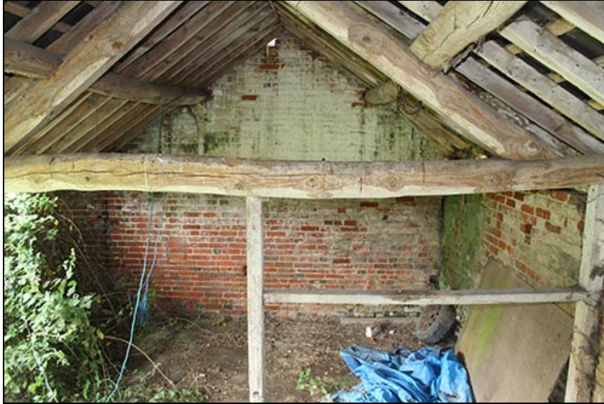
Figure 26 The interior of the Shelter Shed, looking west at the east wall of the Brick Barn
