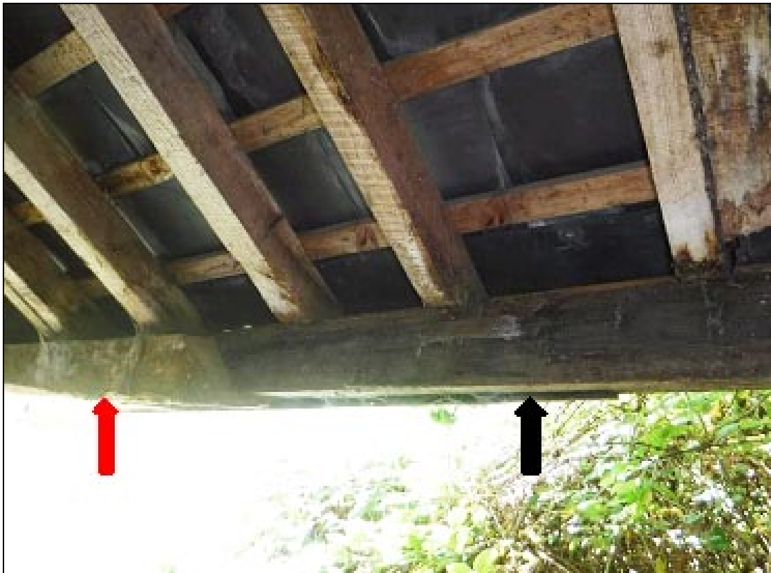
Figure 28 The west end of the front wall-plate of the Shelter Shed, showing the mid-20 th century repair (red arrow) and subsequent early 21 st century repair (black arrow)
