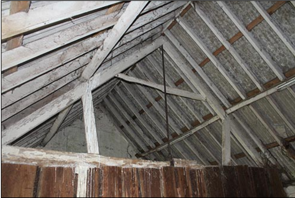
Figure 34 A mid-20 th century roof truss within the rebuilt eastern block of the Stables
