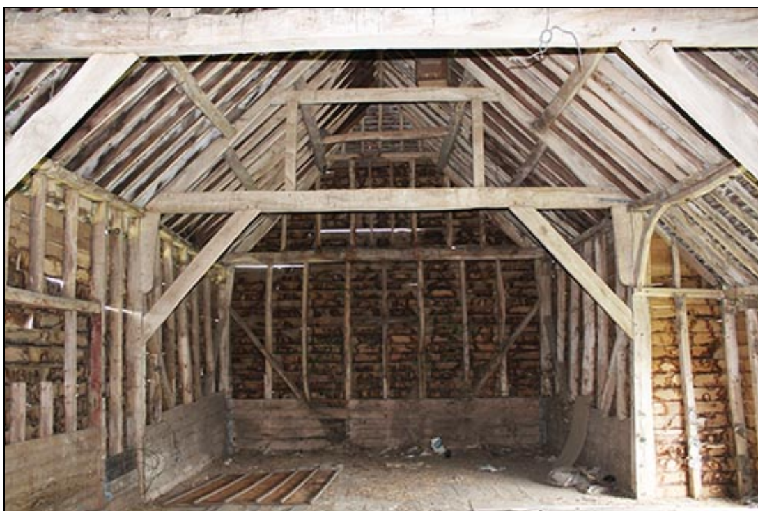
Figure 13 Interior of the Threshing Barn looking west showing the frame construction and the original beech boarding on the lower walls as surviving in the western bay
