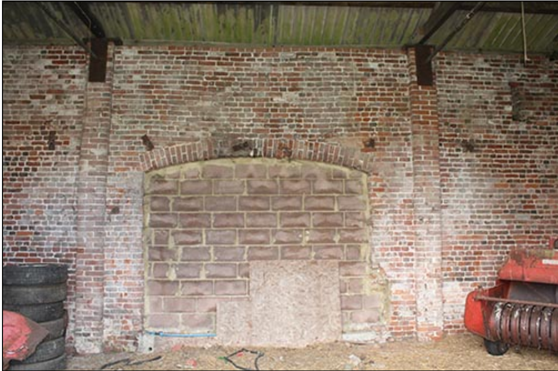
Figure 21 The infilled west door of the brick barn showing the five anchor plates in a row above
