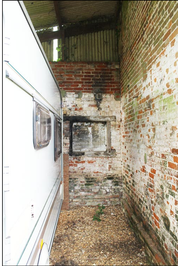
Figure 24 The interior of the Lean-to looking west towards the blocked window in its west wall; above can be seen the infilled sockets for the floor timbers.
