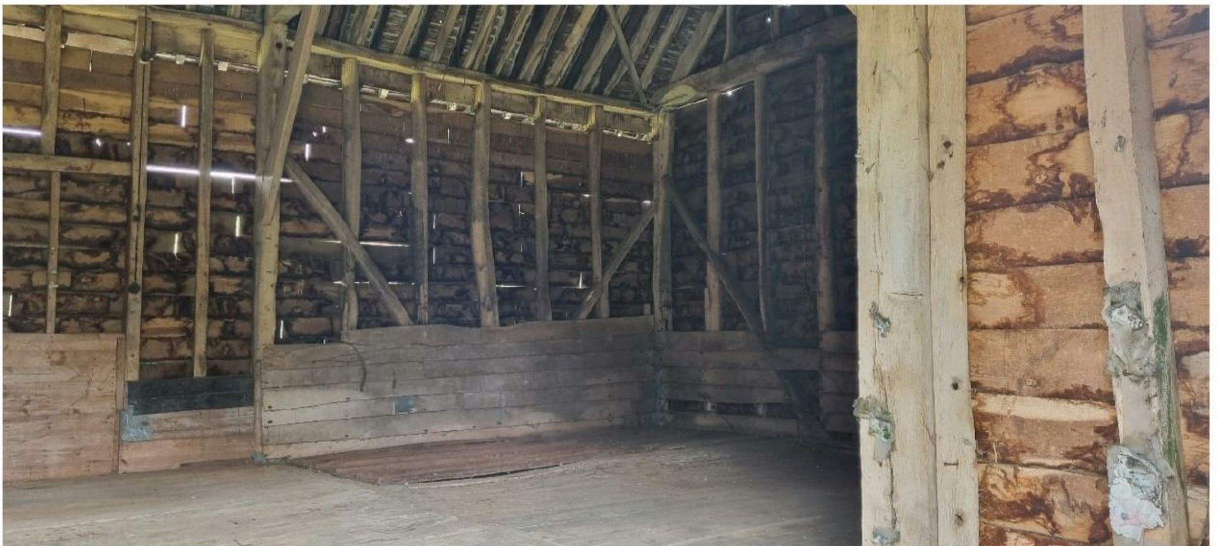
Barn B – Internal structure to be retained, showing areas of cladding and feather boards that require repair.
