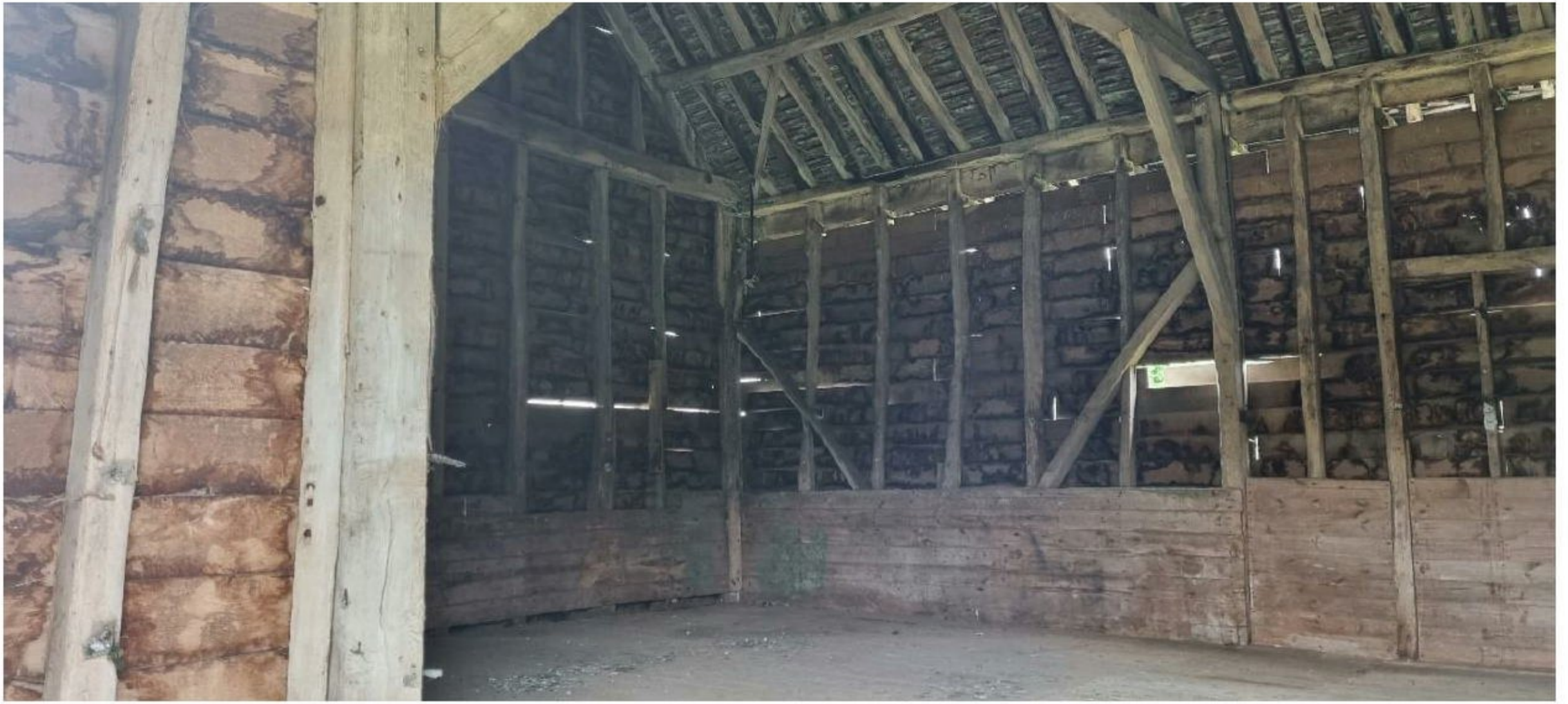
Barn B – Internal structure to be retained, showing areas of cladding that require repair.
