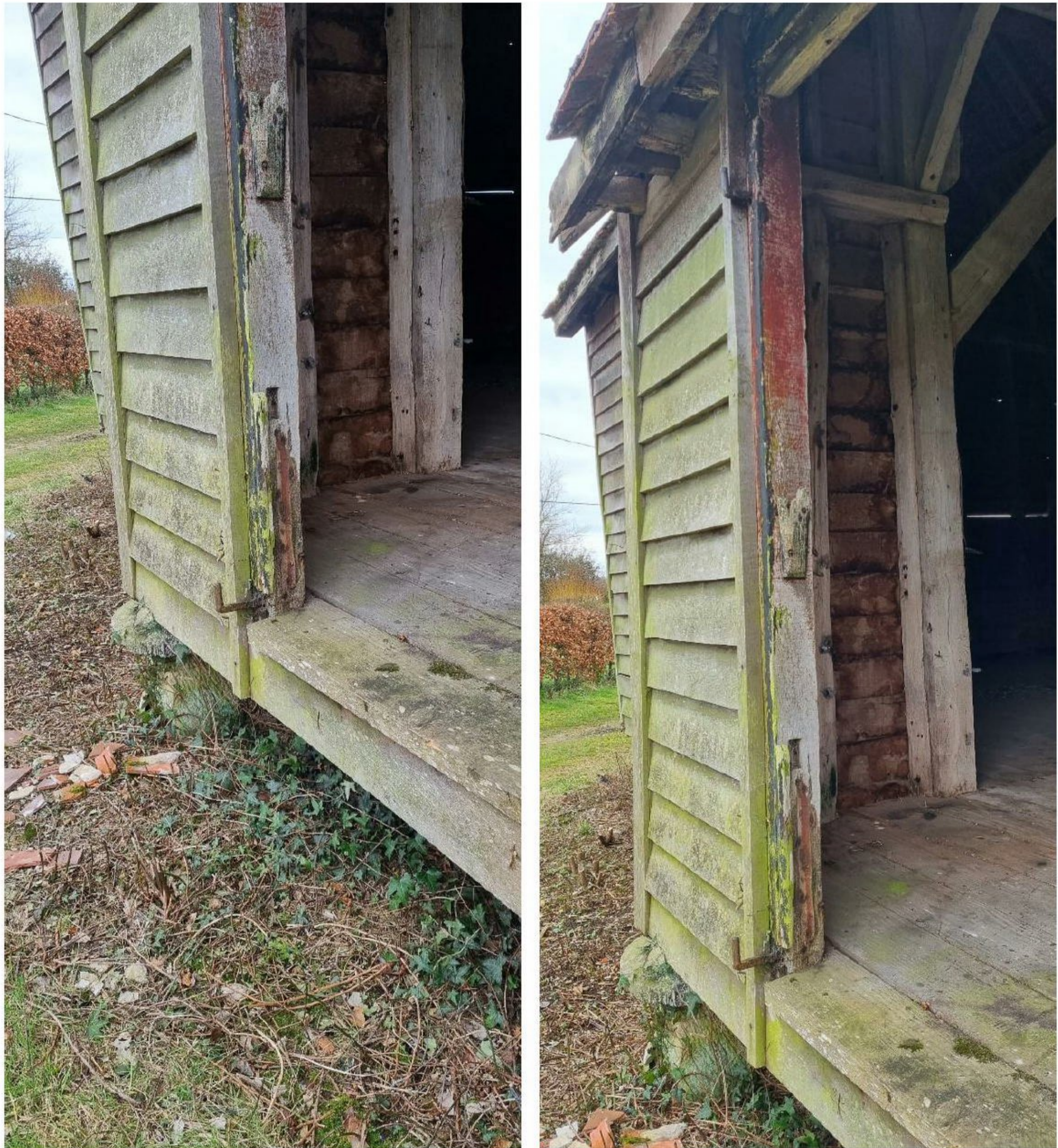
Barn B – Internal structure to be retained, showing existing posts where the glazed screen will be set between.
