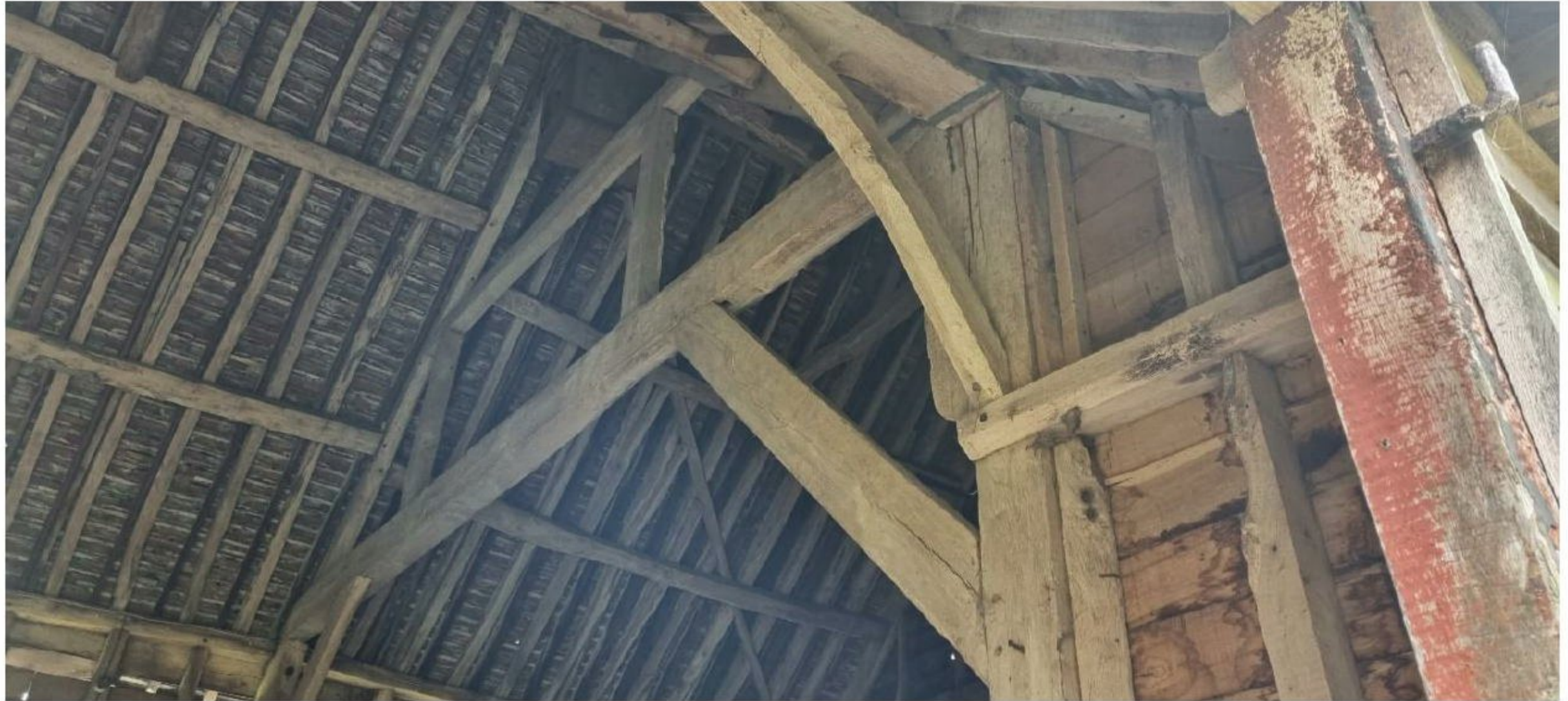
Barn B – Internal structure to be retained, showing existing posts where the glazed screen will be set between.
