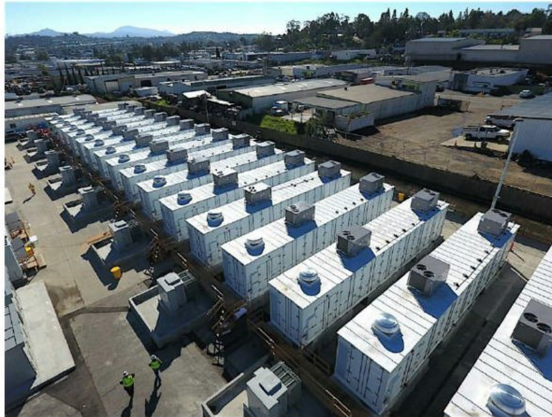
Typical Battery Storage Facility
