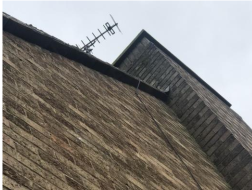
Image 20: B1 viewed from south side. Close-up on lifted lead flashing
