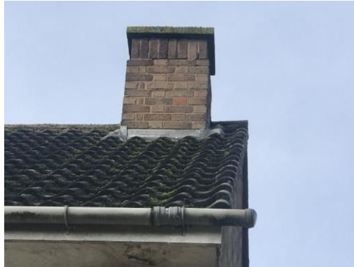
Image 2: B1 viewed from east side. Close up on lifted lead flashing on chimney
