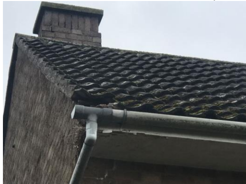
Image 12: B1 viewed from west side. Close-up on lifted tiles
