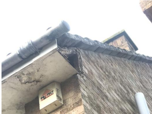
Image 8: B1 viewed from east side. Close up on gap in soffit
