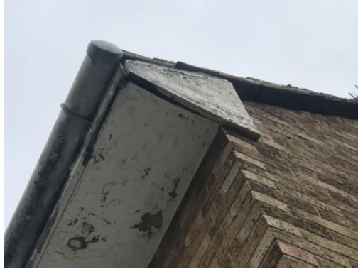
Image 19: B1 viewed from south side. Close-up on gaps in soffits
