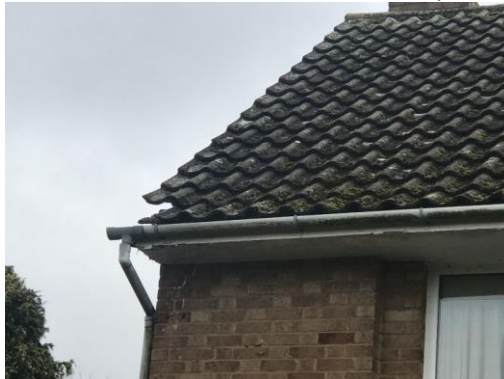
Image 15: B1 viewed from west side. Close-up on lifted tiles
