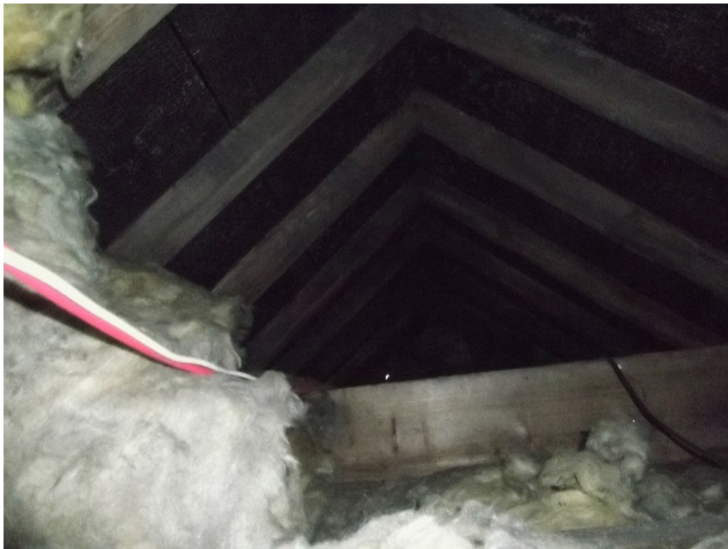
Plate 11. The roof void over the eastern wing viewed from the small pop hole
