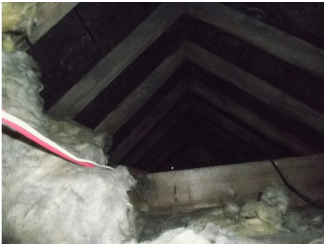
Plate 7. The roof void over the eastern wing viewed from the small pop hole
