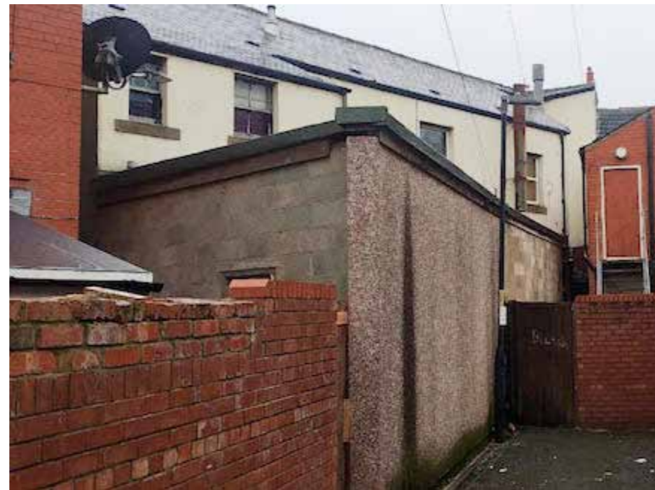
113-119 EGERTON ROAD -REAR ELEVATION FIRST FLOOR (TOWARDS 119 EGERTON RD) FROM ALLEYWAY OFF RICHMOND ROAD
