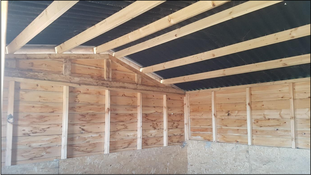
Plate 13: There were no features where bats could conceivably have roosted,. It was possible to search all areas within the sheds.
