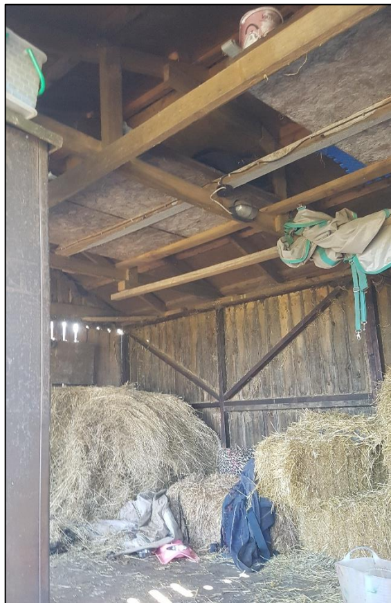
Plate 12: Doors were open and gaps in between wall boards offered bats potentially easy access into the buildings.
