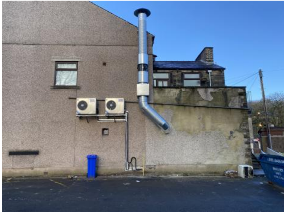
Installed extraction system
