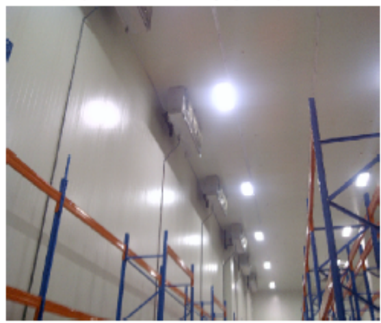
42m long x 12m high ceiling -22C Room, Blower (Evaporator) installation, anti-Freeze LED lamps with back up battery (optional), and heated drains.
