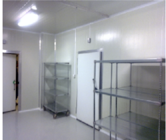
Chiller-Freezer Room, Wall-Floor & Ceiling seamless monolithic finish with alarm system system above freezer heated door (optional)
