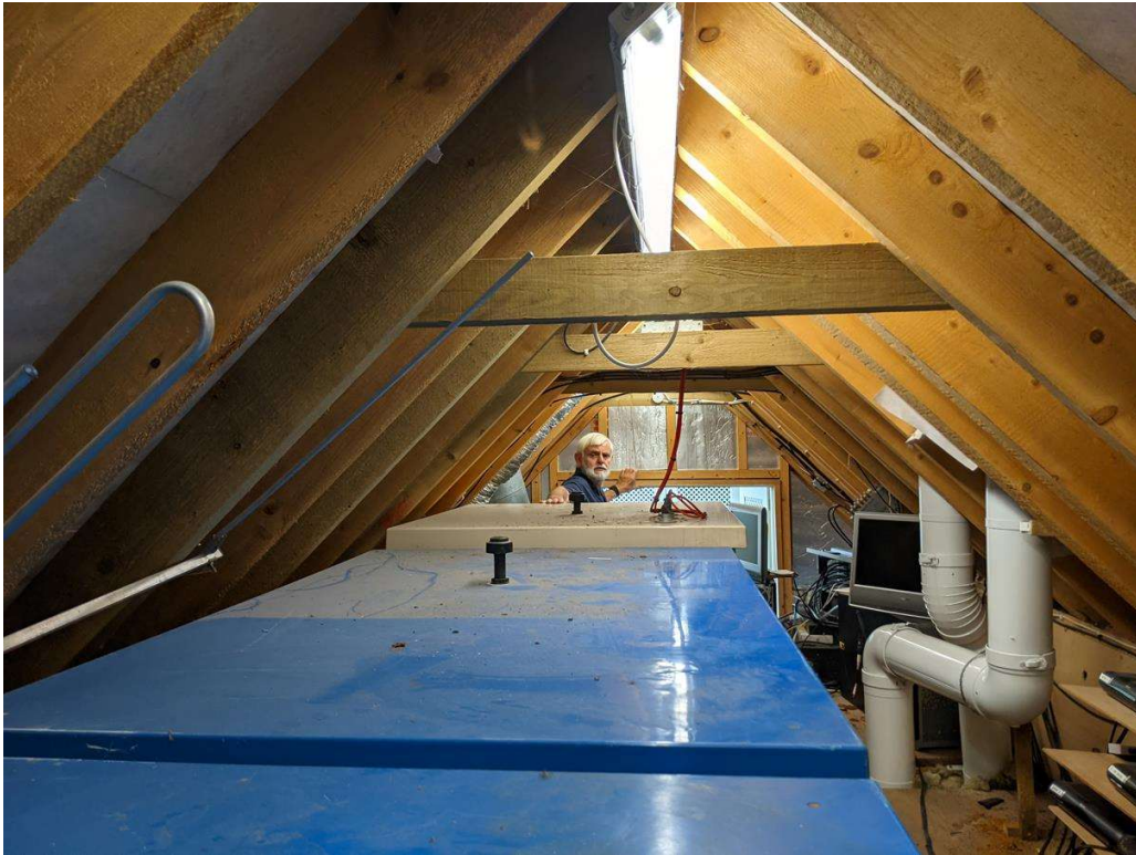
Photograph No. 03 – View of loft of small roof of section 1 of B01.
