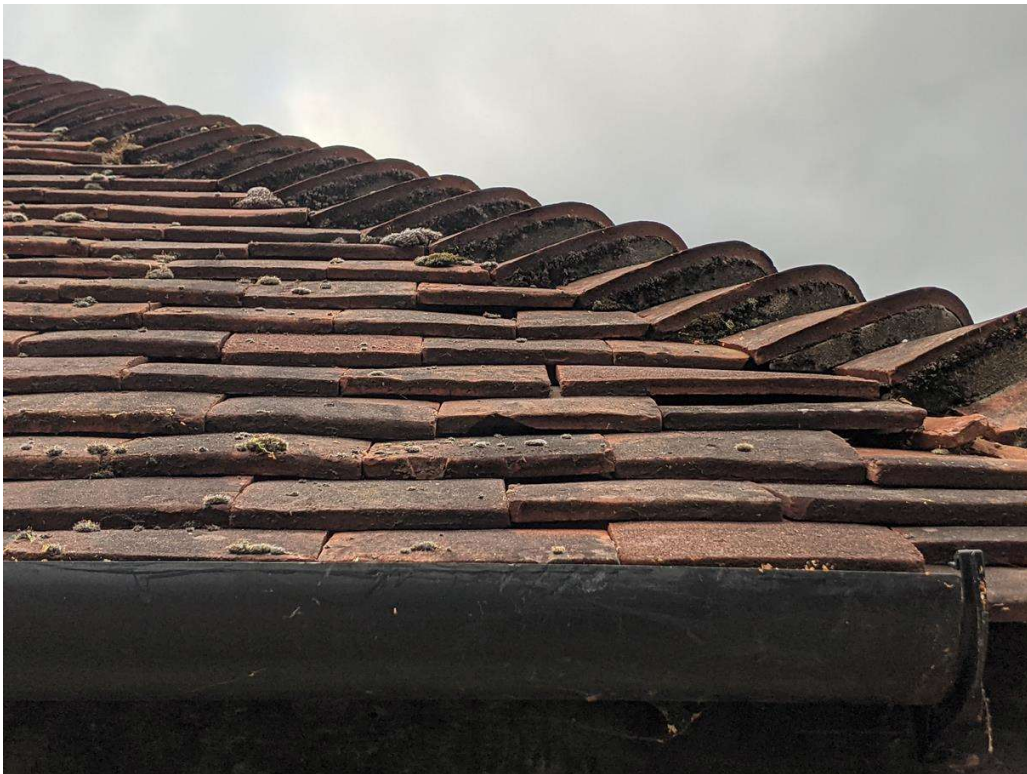
Photograph No. 12 – Lifted tiles to B03 Baytree cottage.
