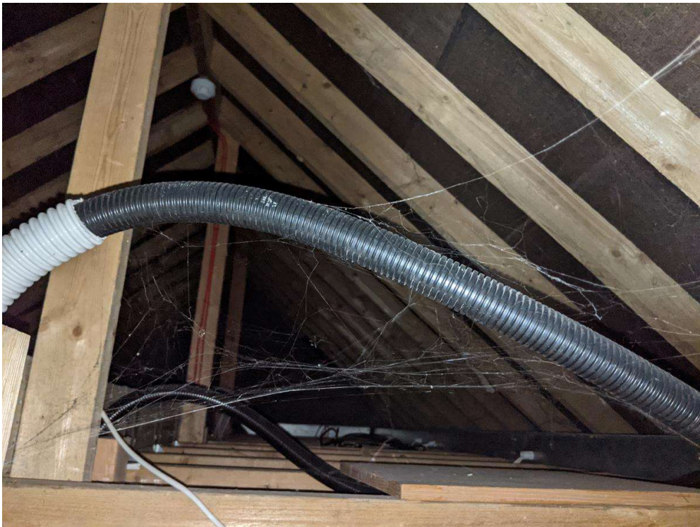
Photograph No. 08 – Cobwebbed loft of B02.
