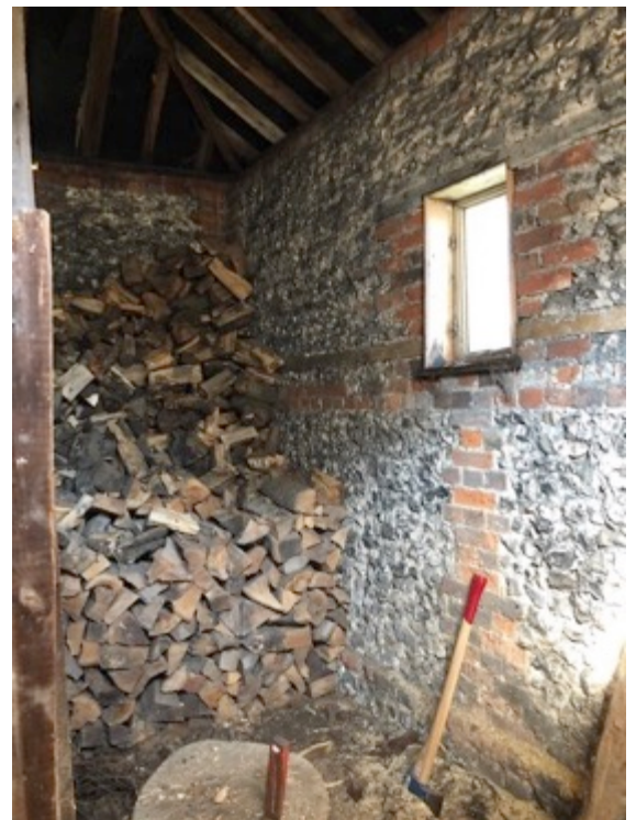
10 Log Store at north end of the building, showing crude nature of wall finish and exposed roof structure.
