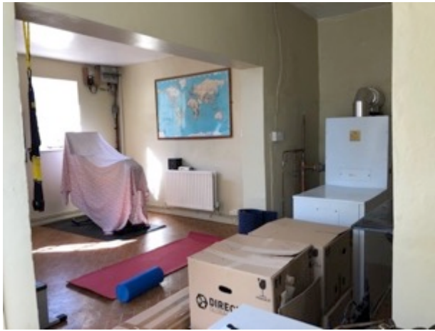
7 Fitness Room, viewed from old Tack Room. The boiler shows on the right.
