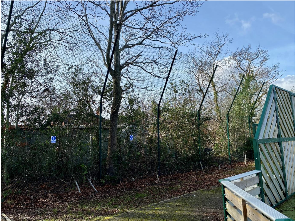
Picture showing current cantilever ball retention fence on far boundary. This will be relocated on the newly erected 3m green mesh fence.
