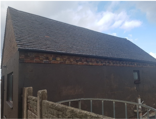
D: Part Side View of Existing Stable Unit
