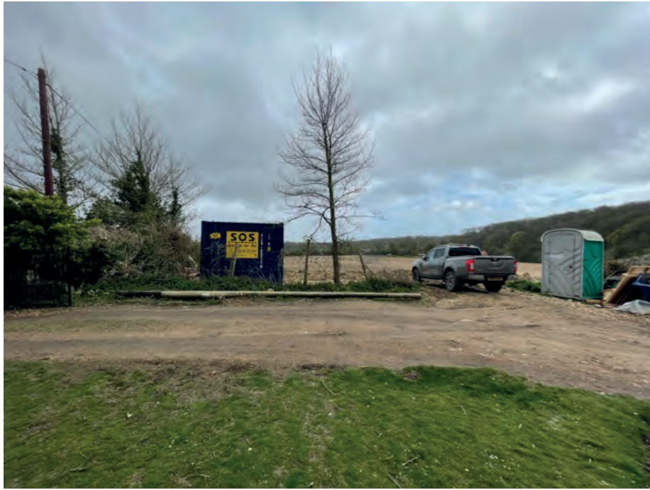
The Builders for the kitchen are currently using the site as a storage area for the Kitchen Project.
