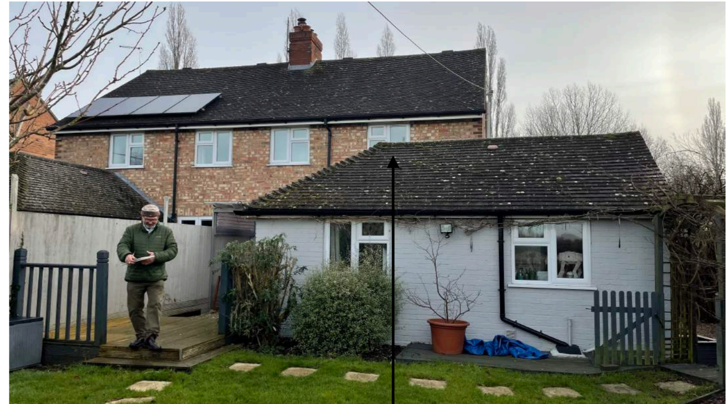
Two storey extension proposed to go erected above existing single storey utilities and office room shown here.
