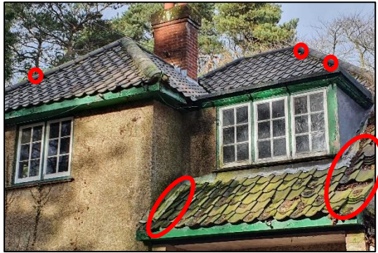
Figure 3: Southern aspect – gaps circled.
