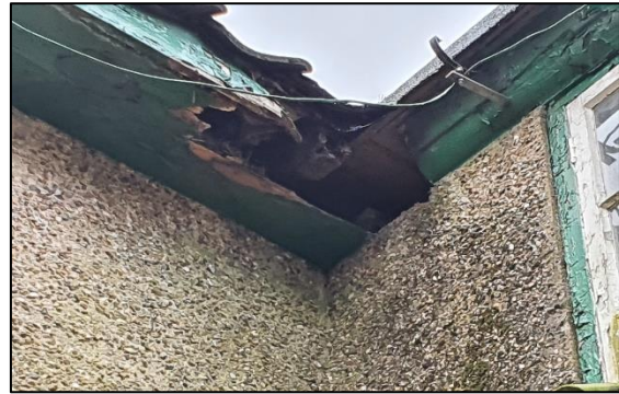
Figure 4: Gap in otherwise well-sealed soffit
