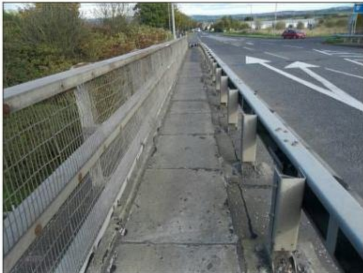
Photo 2.12 – Northern footway along the M90 overbridge looking eastwards towards the M90 southbound off slip
