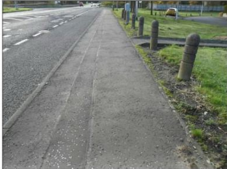
Photo 2.15 – Northern footway along the A909 Cocklaw Street looking westwards towards the M90 Junction 4 interchange
