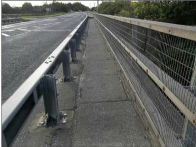
Photo 2.11 – Northern footway along the M90 overbridge looking westwards towards the M90 northbound on slip
