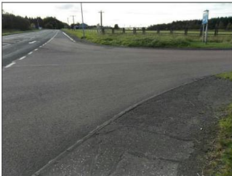
Photo 2.9 – Northern footway from the M90 overbridge looking westwards across the M90 northbound on slip
