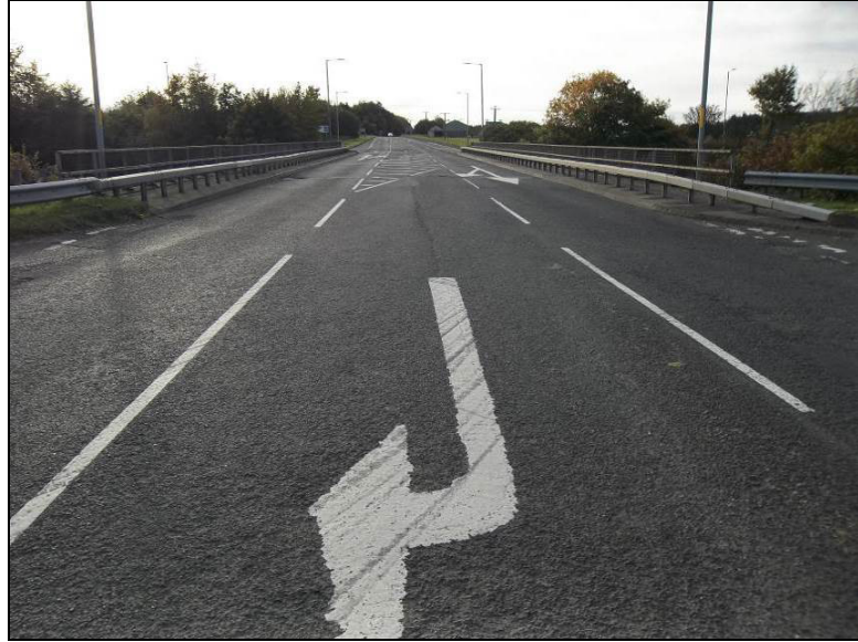
Photo 2.35 – A909 looking westwards with the right turn lane for the M90 southbound on slip
