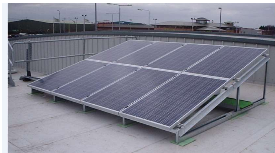
Typical PV panel installation
