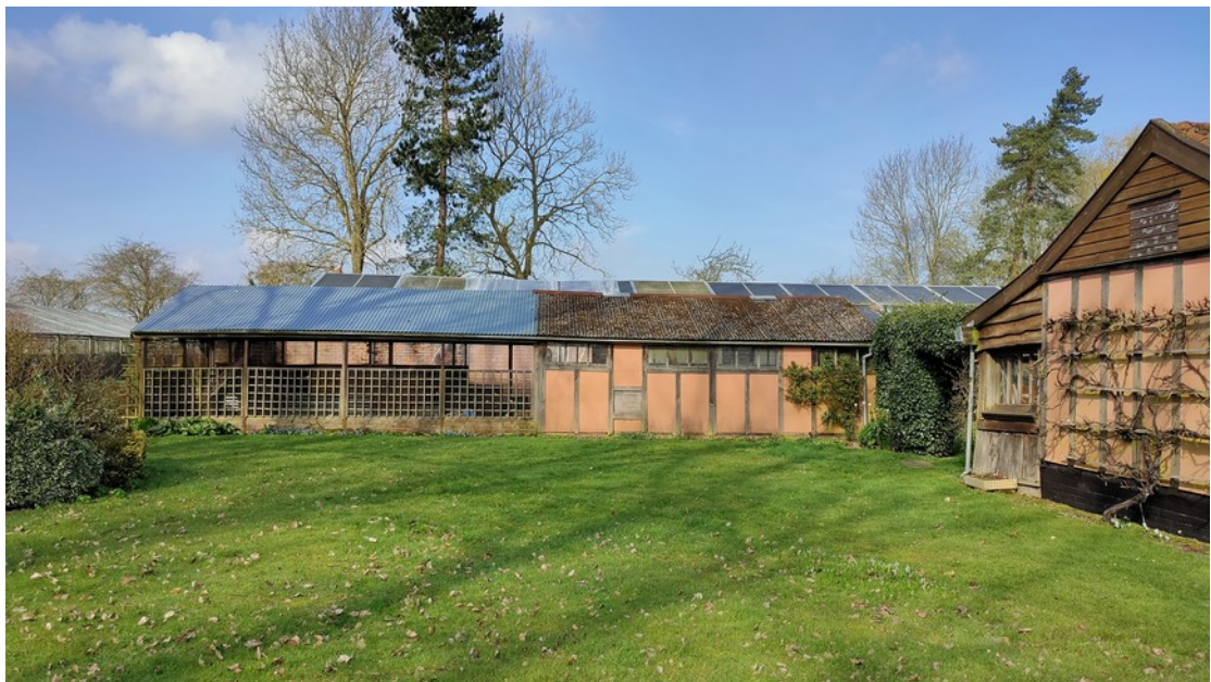
Outbuilding. LH section to be removed and RH to be clad in weatherboarding. Roof replaced with set aside metal roof over potting shed element.
