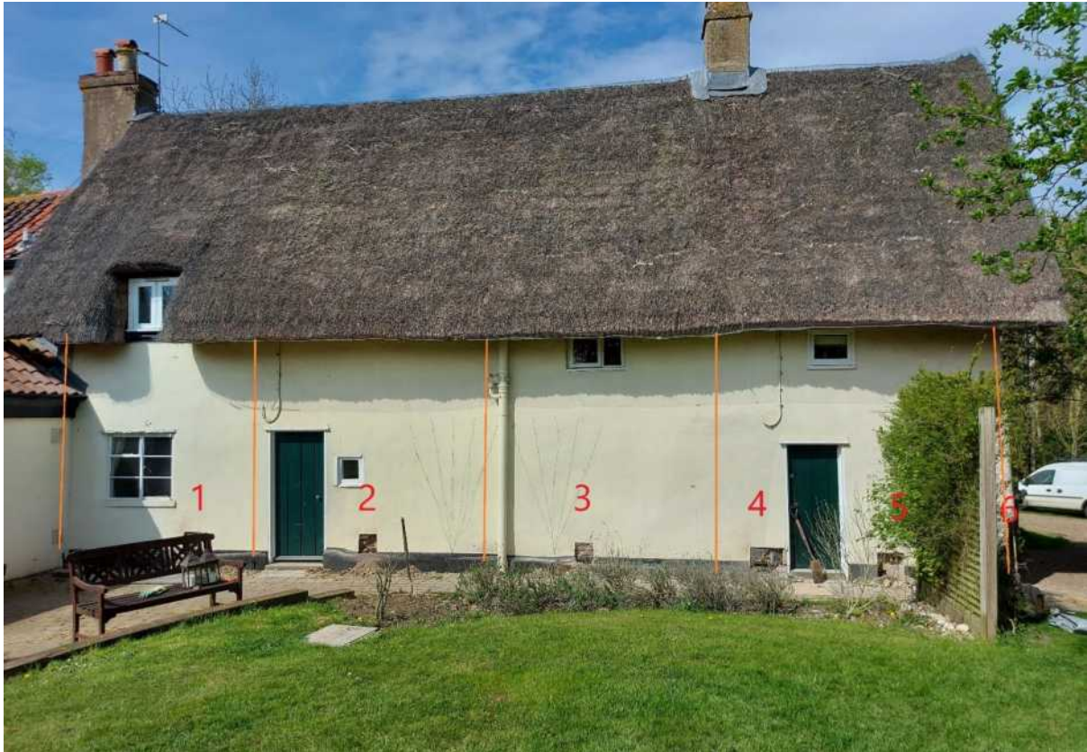
Above, the south elevation with six sections of render removed and crossframes marked in orange.
