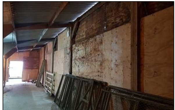
Figure 5: Light coming through the gap between the roof and the walls.
