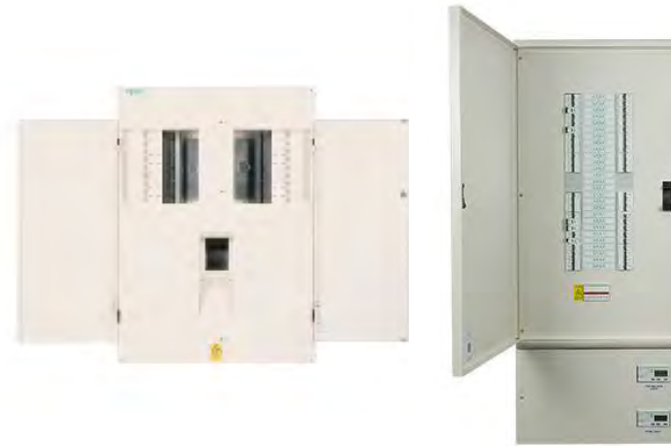
Figure 9.5.1: Typical examples of panel boards (left) and final circuit distribution boards (right) for Landlord system use.
