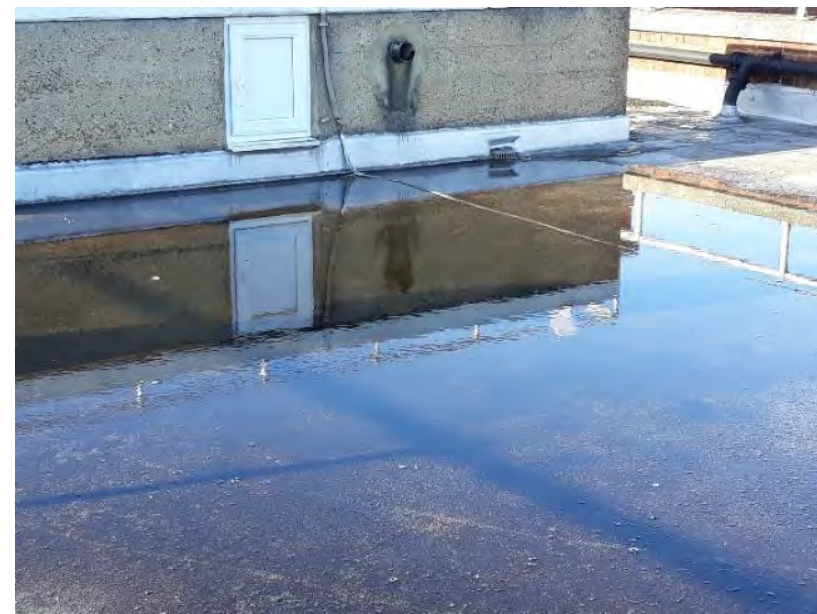
Figure 8.4.2 existing roof area with ponding
