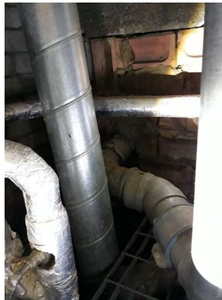
Figure 8.3.1 Typical apartment service riser installation
