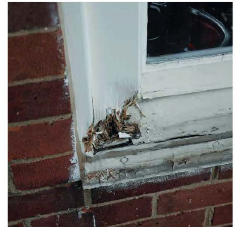
Example of existing window degrading
