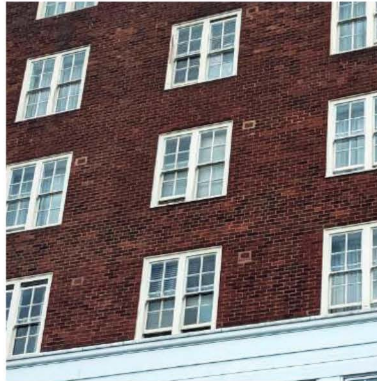
Air bricks on Chichester Street show poor workmanship
