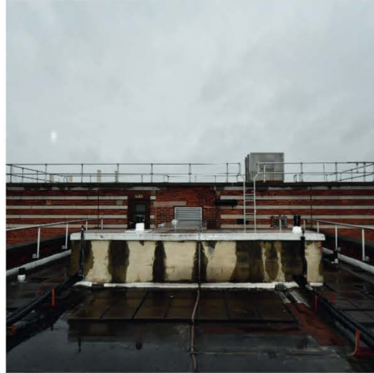
Typical roof environment - Services compartment
