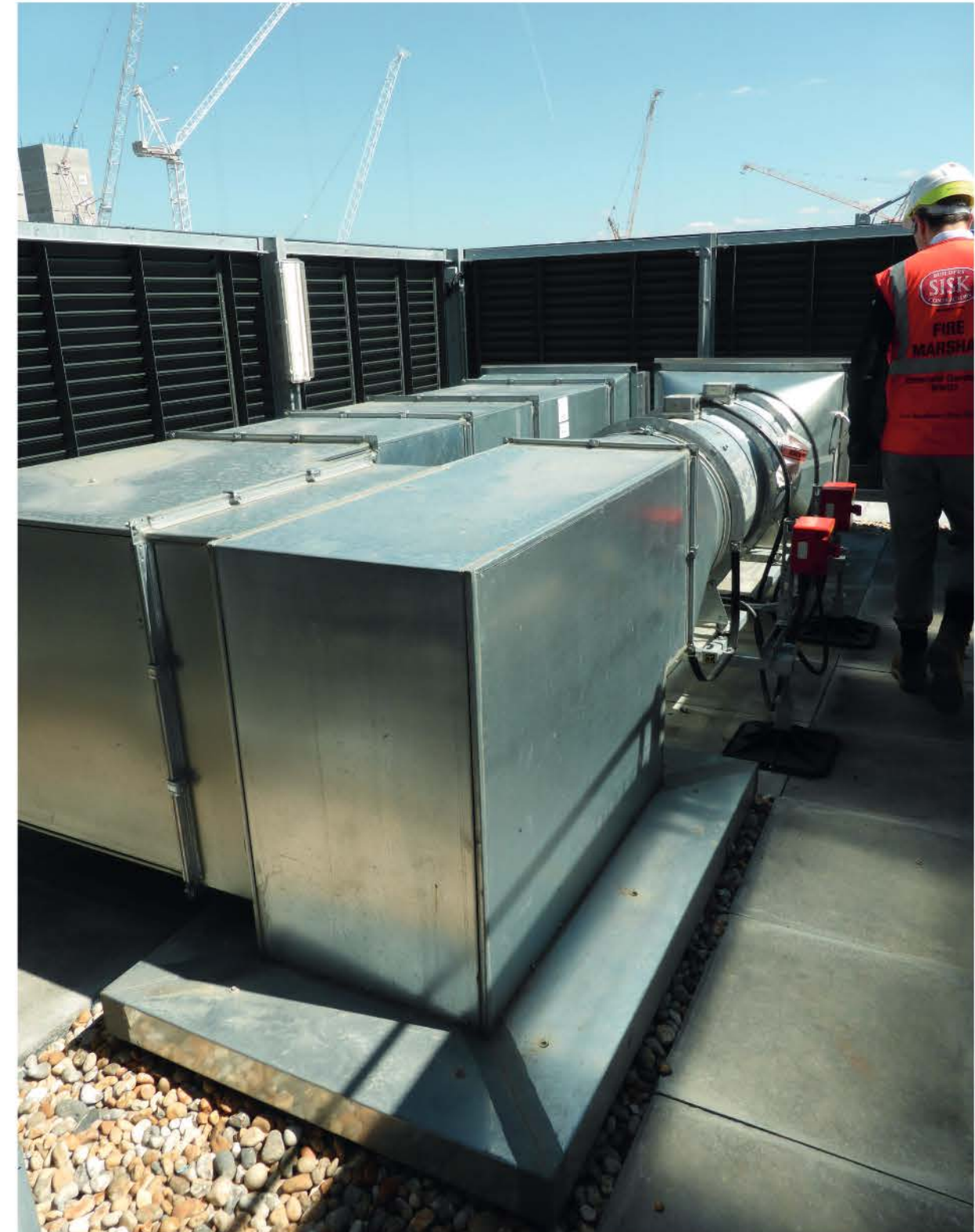
Smoke Extract Fans within Enclosure
