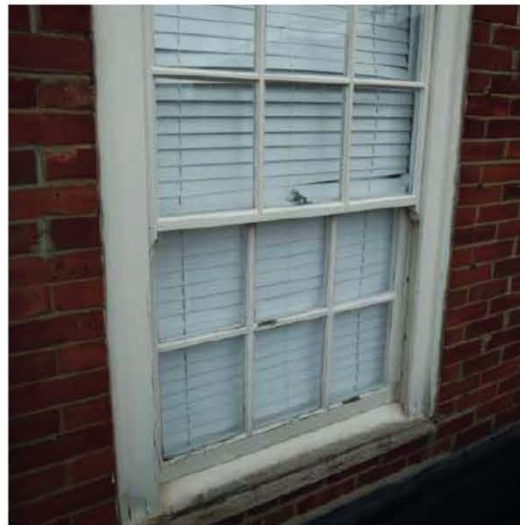
Example of existing window degrading
