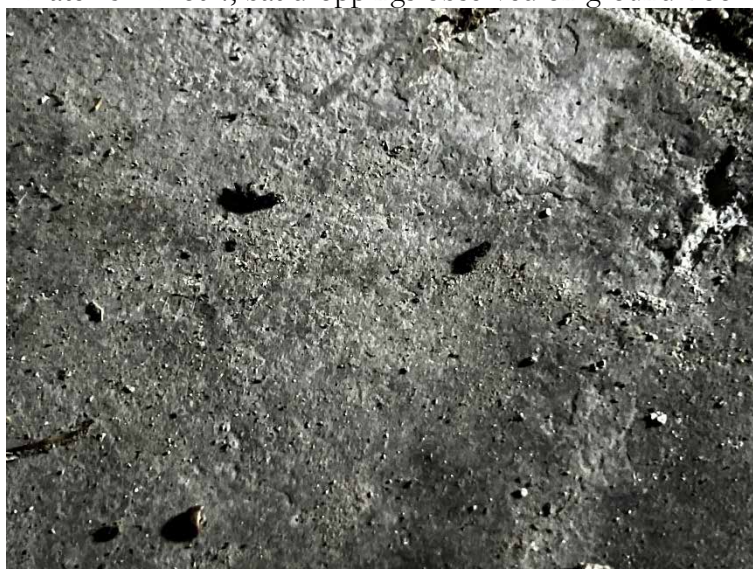
Plate 15 – Plot 4, bat droppings observed on ground floor
