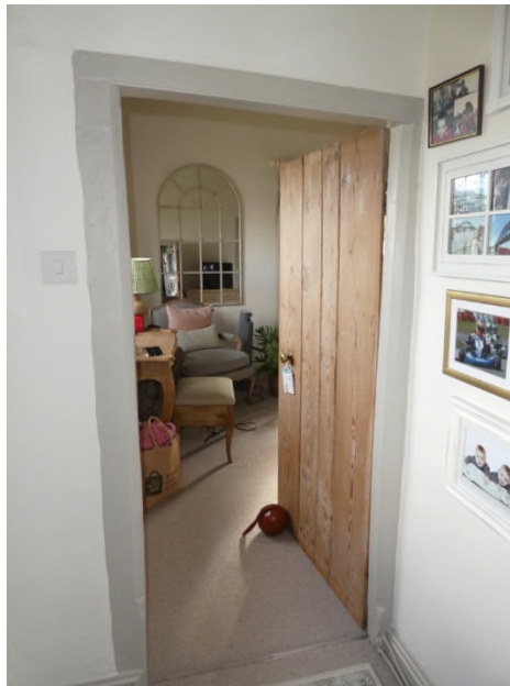
Figure 16: Plank and batten door and chamfered door frame to the first floor bedroom
