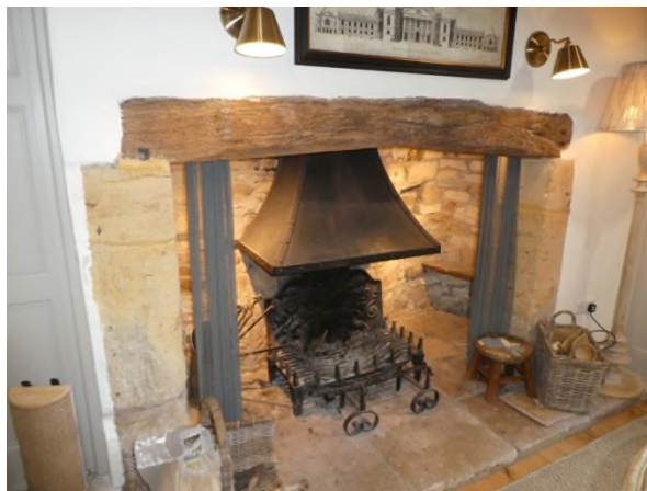
Figure 9: Fireplace with stone jambs and a timber lintel with chamfer and stop details
