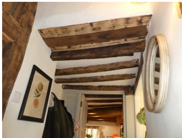
Figure 15: Timber lintel and joists on the south-west side of the chimney breast
