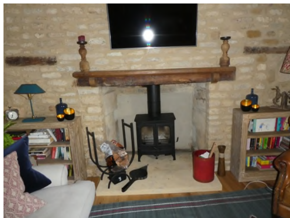
Figure 27: Fireplace with a timber lintel and blocked openings with lintels to the left and right
