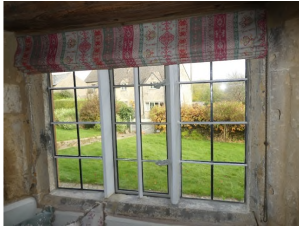
Figure 11: 3-light window with narrow chamfered mullions and a 19 th century iron casement
