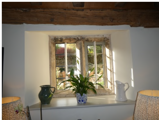
Figure 10: 2-light window with chamfered mullions and a 17 th to early 18 th century iron casement
