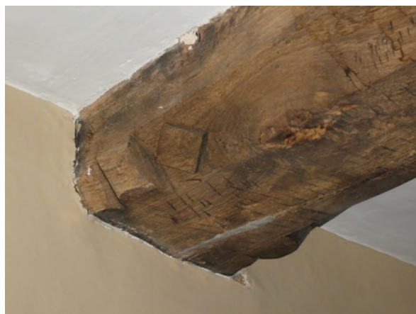
Figure 26: Detail of the transverse beam with bar and scroll stops with lozenge
