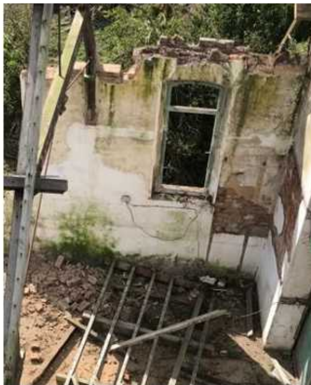
Figure 5: The damaged caused to the original building.
