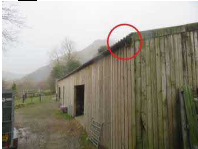
No downpipe connected to front gutter
