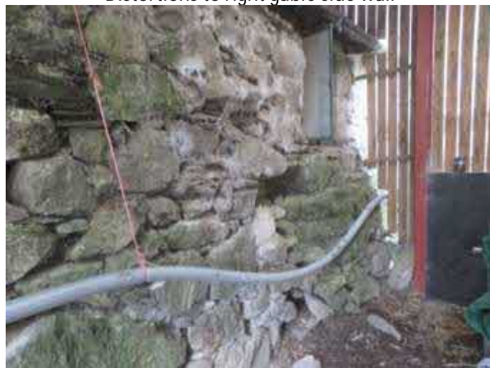
Distortion at bottom corner
