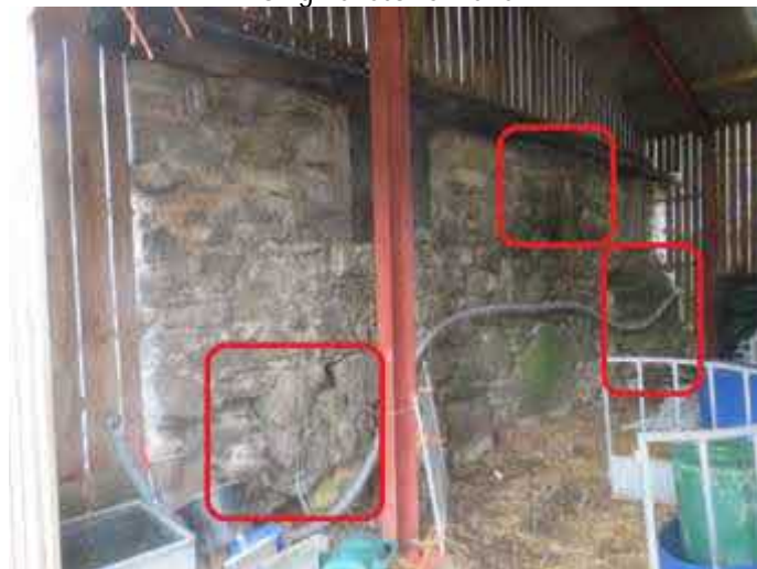
Distortions to right gable side wall
