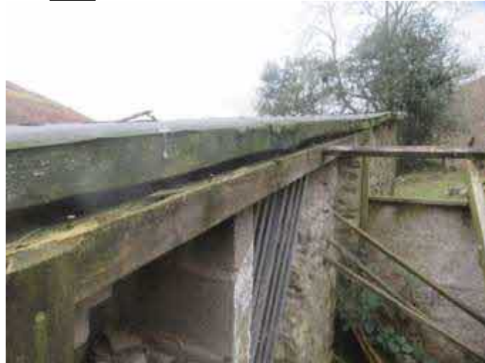
Deterioration to bargeboard timber
