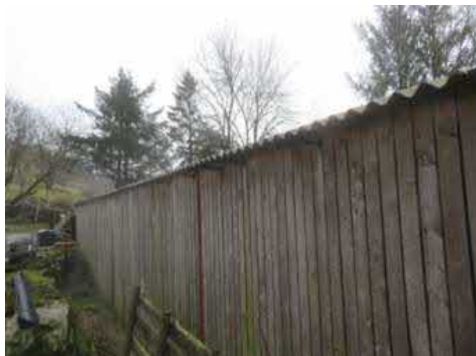
Missing gutter to rear roofline
