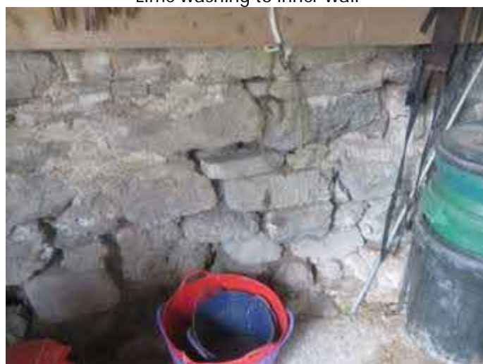
Inner distortions to stone walls
