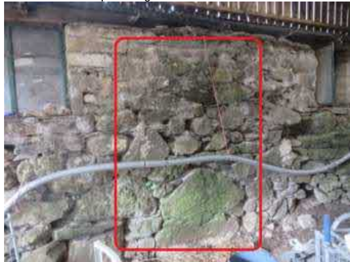
Green 'biological growth' staining
