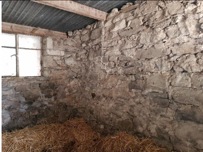
Internal stonework is mostly well-sealed with cement. Some surface gaps present.
