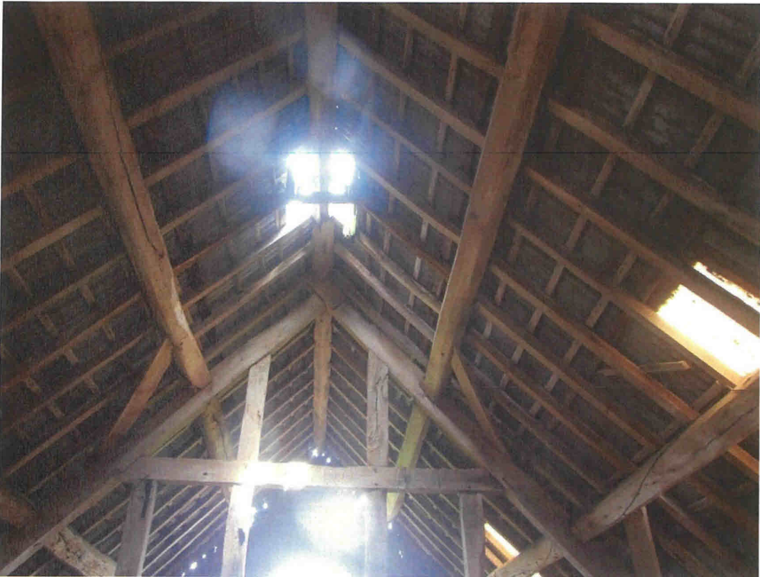
Barn B internal first floor showing truss configuration central and right side.
