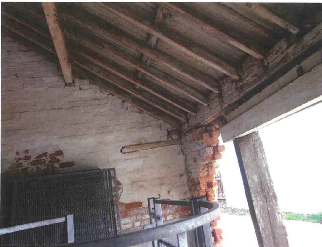
Barn A impact damage to single story.
