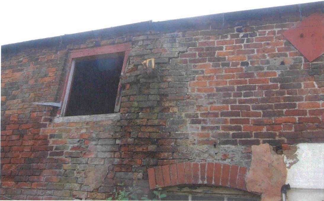
Barn A showing self-seeded tree and damage.
