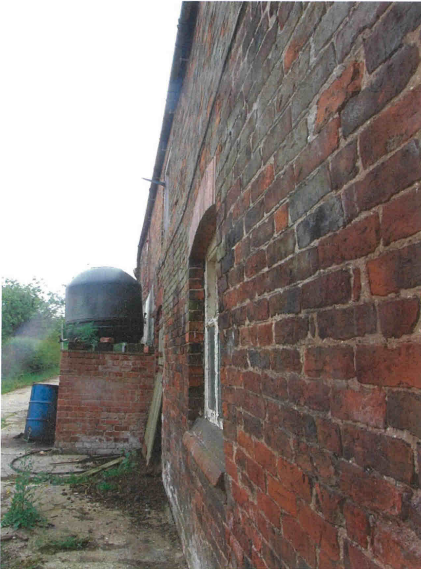
Barn A front elevation, showing undulation due to self-seeded tree and some loss of lateral restraint.
