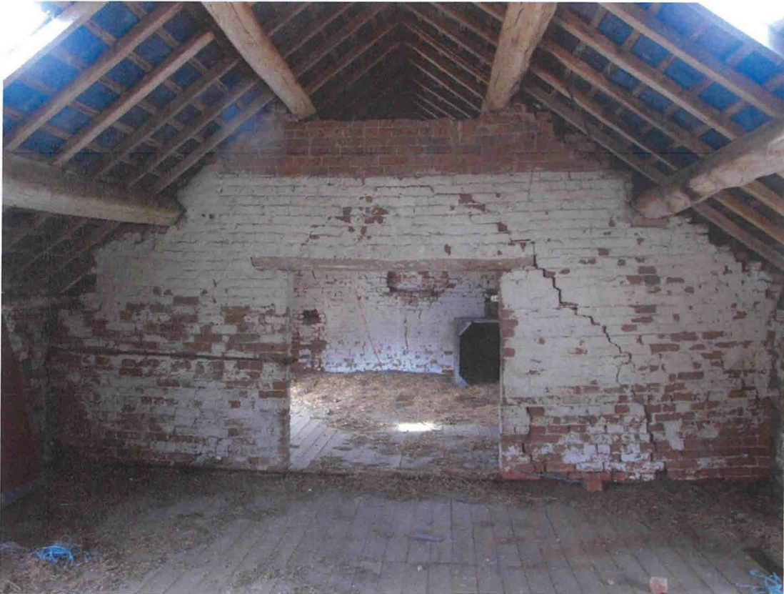
Barn A first floor, minor cracking due to deflected beam.
