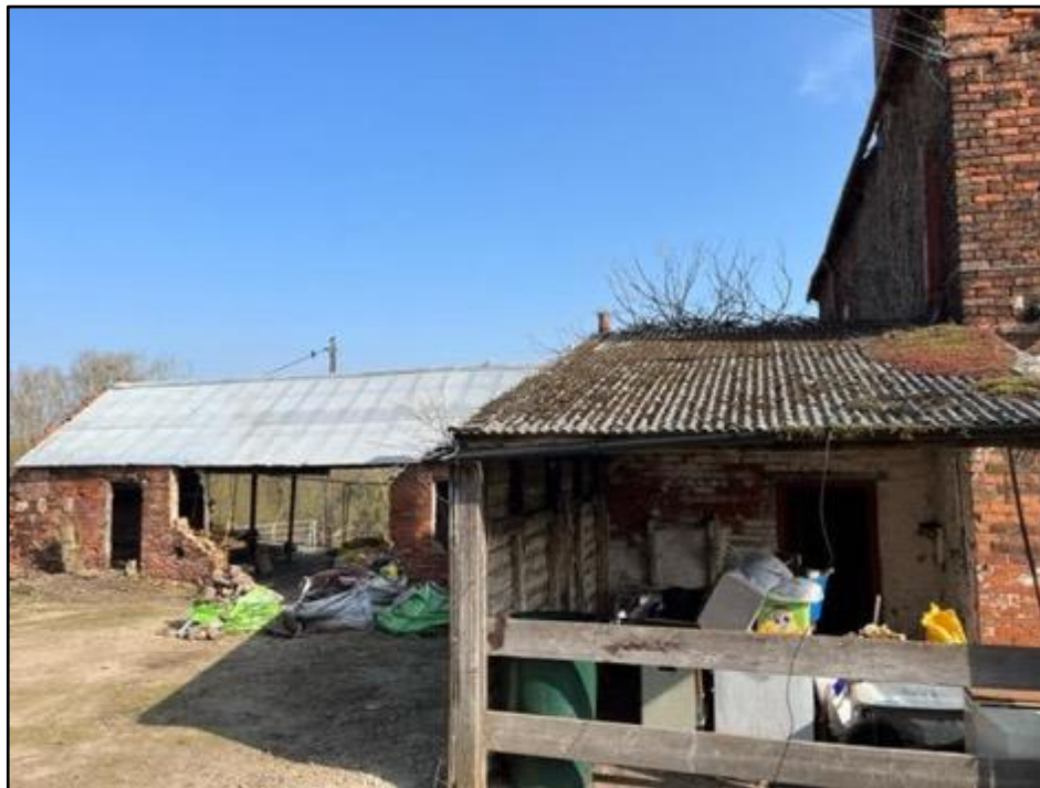
Fig 7: A single-storey extension on the western side of the building. Both this extension and the outbuilding feature a tin roof atop; this roof type is unsuitable for bird species and bats.
