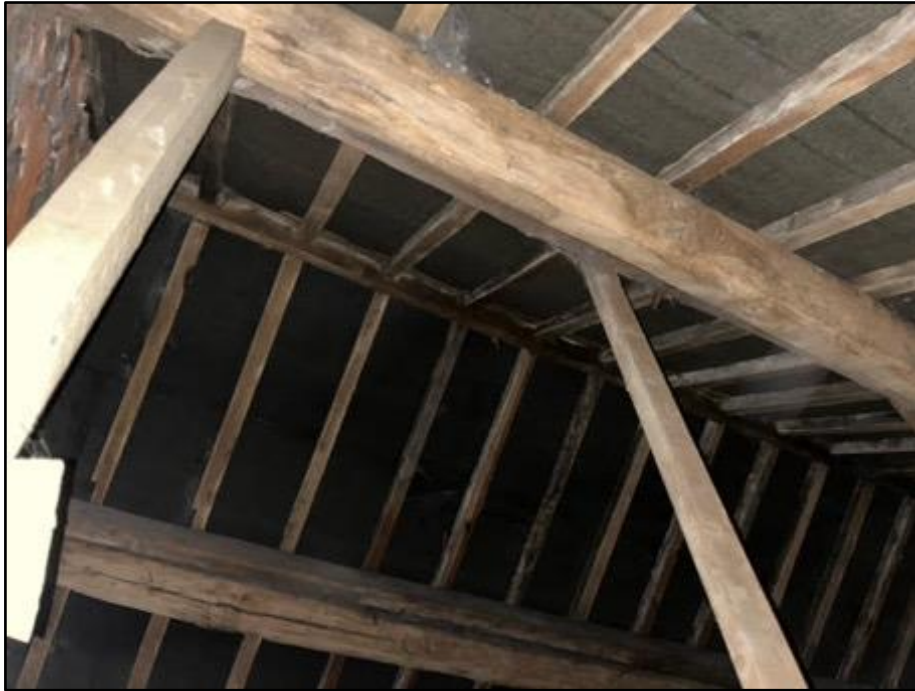
Fig 8: The internal roof space of the building. A felt lining beneath the slate tiles is in fair condition.
