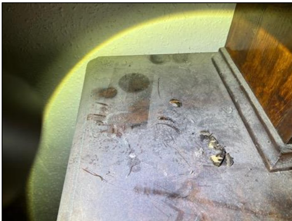
Fig 11: Feeding remains found on the second storey of the building.
