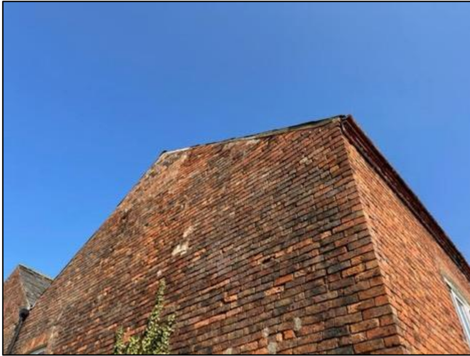
Fig 4: The southern gable is more conditioned than the northern face. The brick soffit of the building is damaged in parts.
