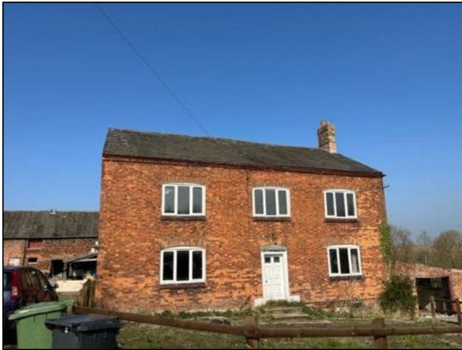
Fig 2: A front view of the subject farmhouse. The roof can be seen in fair condition with several entry points along the apex.
