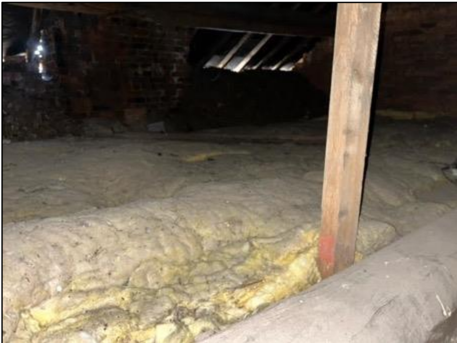
Fig 9: The extent of the roof space. House sparrows and jackdaw nests were identified within the roof space.
