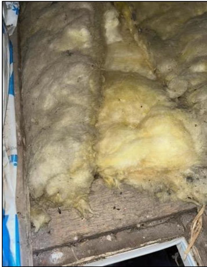
Fig 10: Bat droppings found within the roof space.
