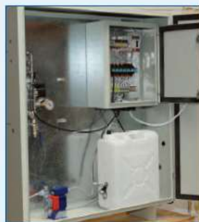
INTERIOR OF AUTOWASH CABINET
