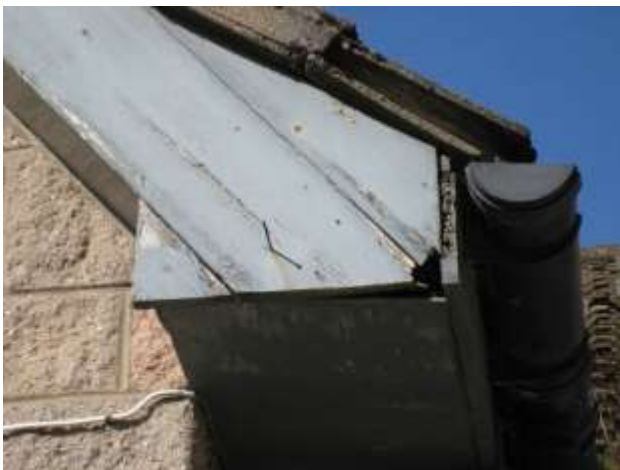
Photo 15: Rot hole in soffit box.
