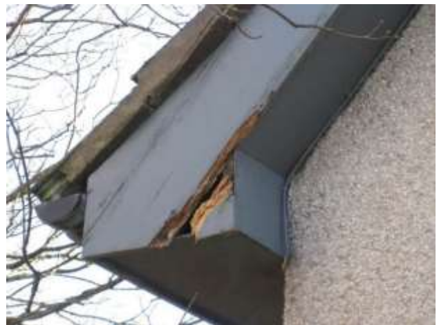
Photo 16: Rot hole in soffit box and gaps between the soffit box and roof tiles.
