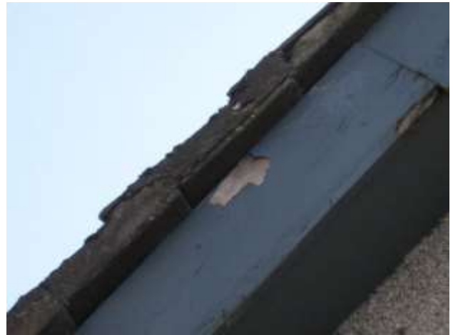
Photo 14: Gaps between the soffit box and roof tiles.
