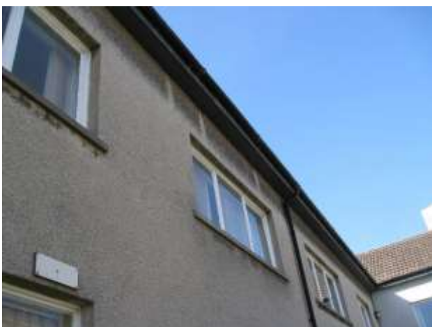
Photo 17: Gaps where the soffit box meets the wall.
