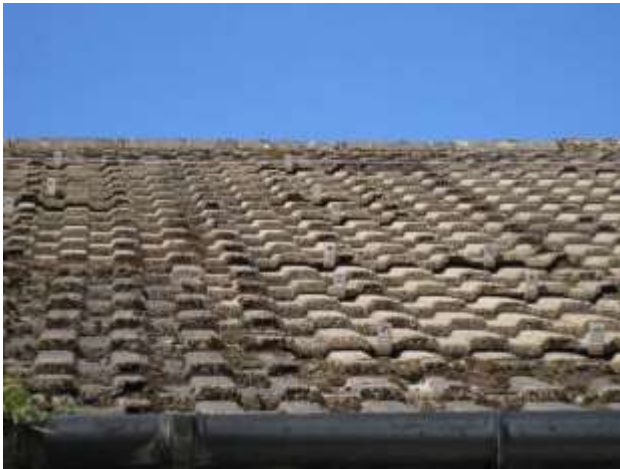
Photo 13: Gaps under the concrete roof tiles.
