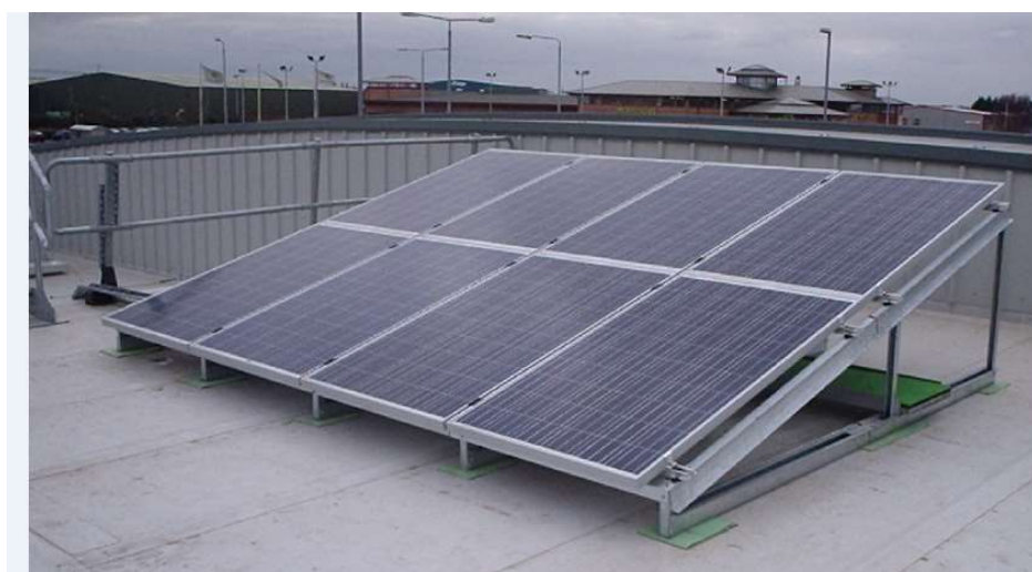
Typical PV panel installation
