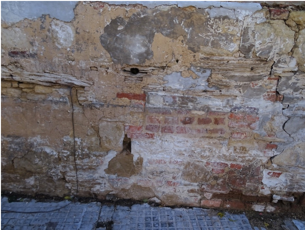
Photograph 9: Building 3 gaps in timber and brickwork of interior wall
