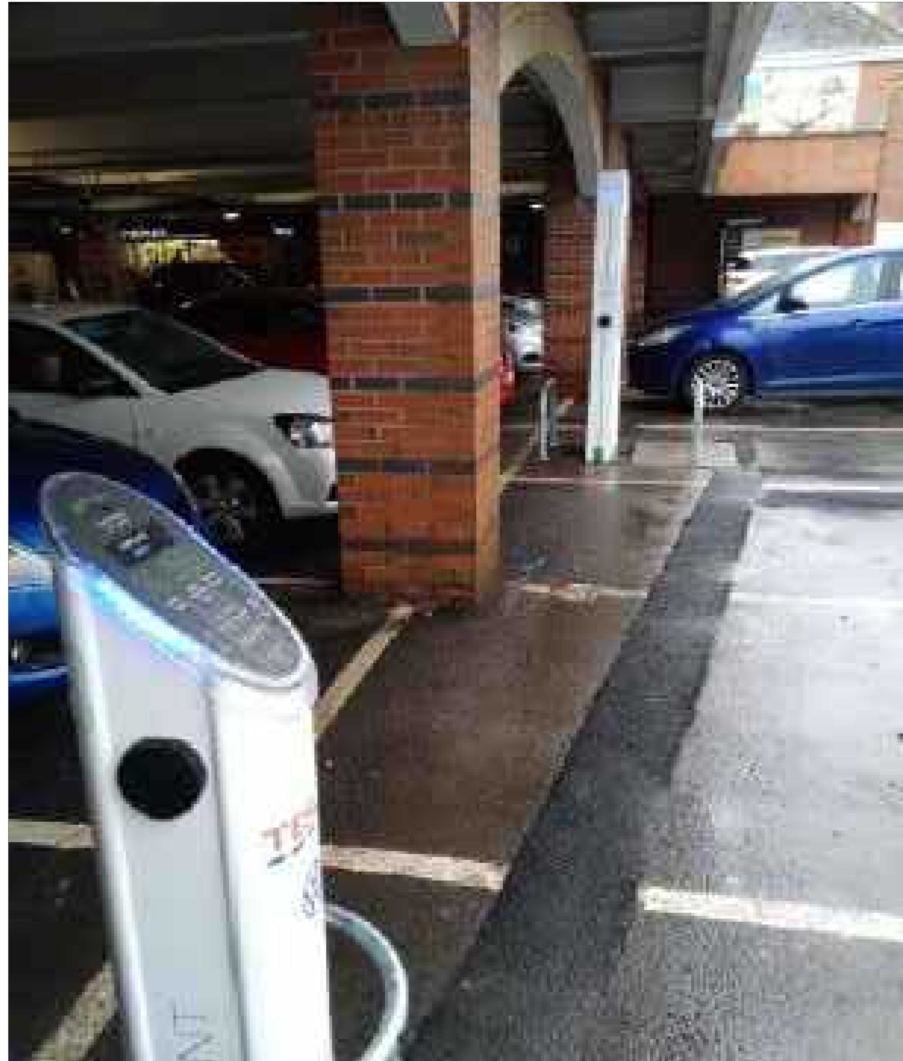
ELECTRIC VEHICLE-CHARGING AREA AT SITE
