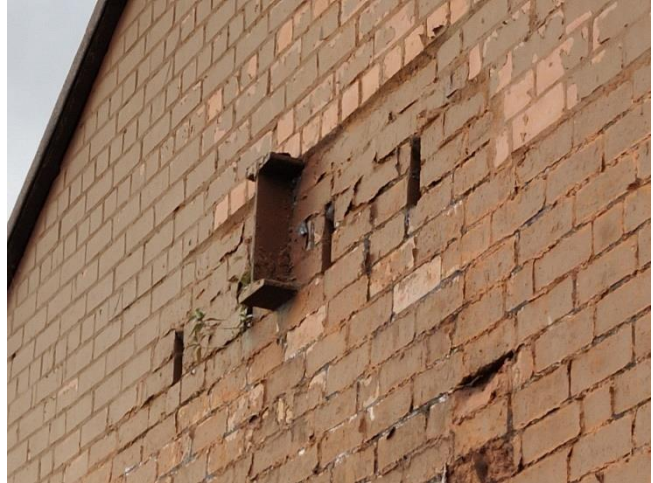
Photo 18: Gaps between bricks at the south elevation of B3.
