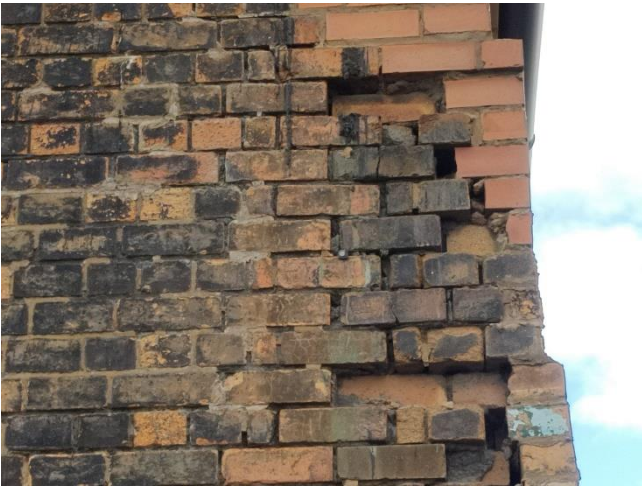
Photo 19: Missing mortar between bricks at the north elevation of B3.
