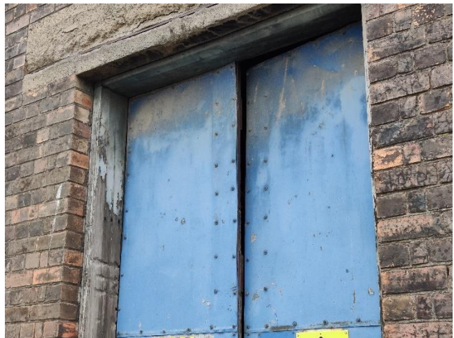
Photo 16: Gap in the door at the north elevation of B3.
