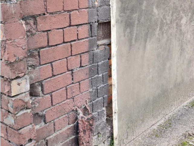
Photo 17: Gap behind plastic sheet at the east elevation of B3.
