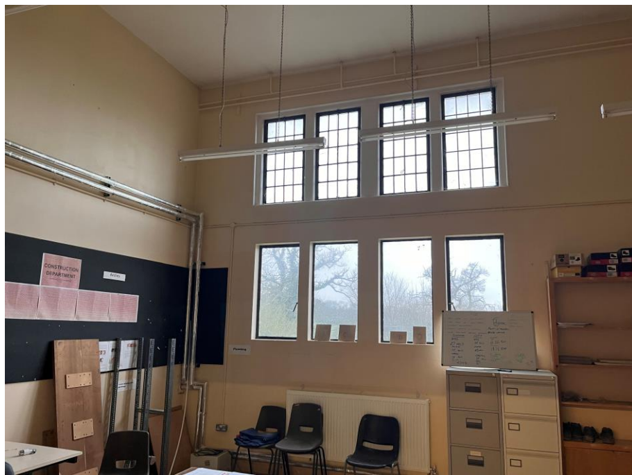
Figure 18: Photograph of the northern most room which has already been altered in character through dry lining of the walls and introduction of a replacement floor
