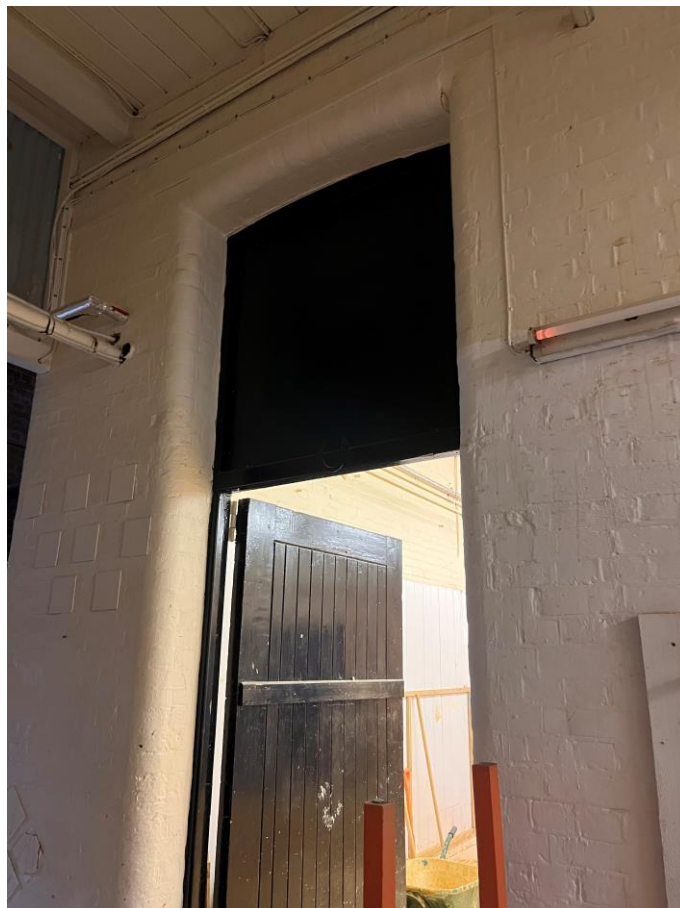
Figure 24: Existing door leading from the lobby into the southern room with currently blocked fanlight above
