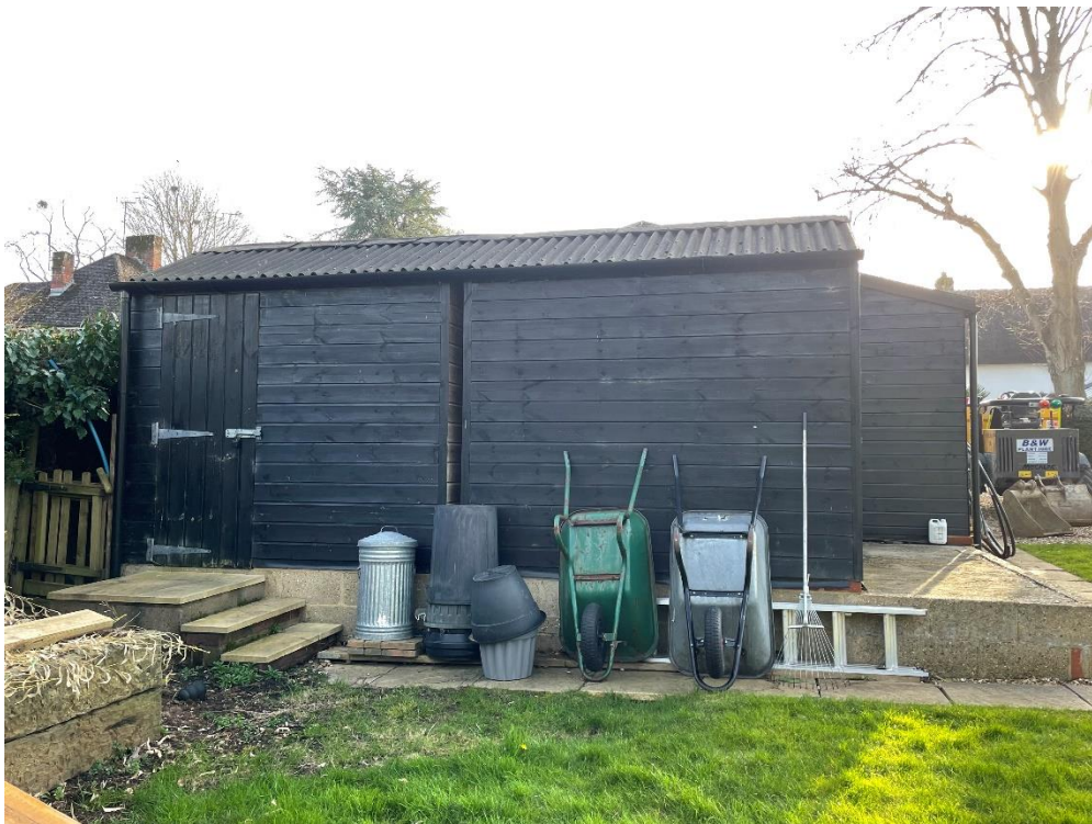
Front elevation facing down the garden, away from the house and the street.
