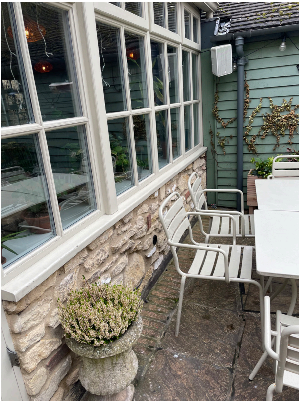
Fig.2.5 View of coarsed rubble limestone wall and timber painted windows to Courtyard.
