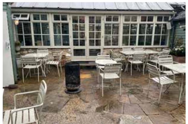
Fig. 2.6 View of coarsed rouble limestone wall and timber painted windows to Courtyard.
