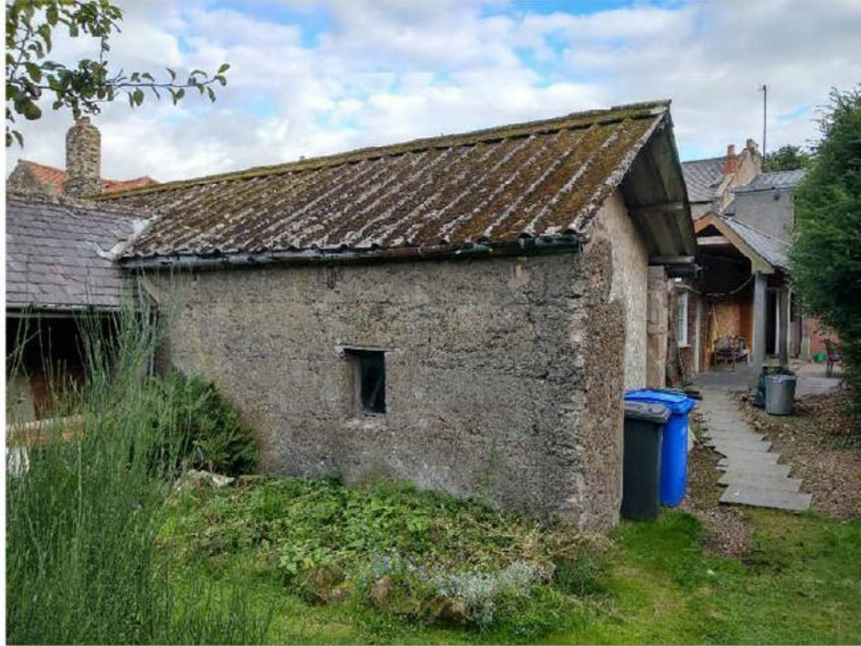
The Old Cowshed is built of poor shuttered concrete under an asbestos roof. It is not capable of conversion so is to be replaced.
