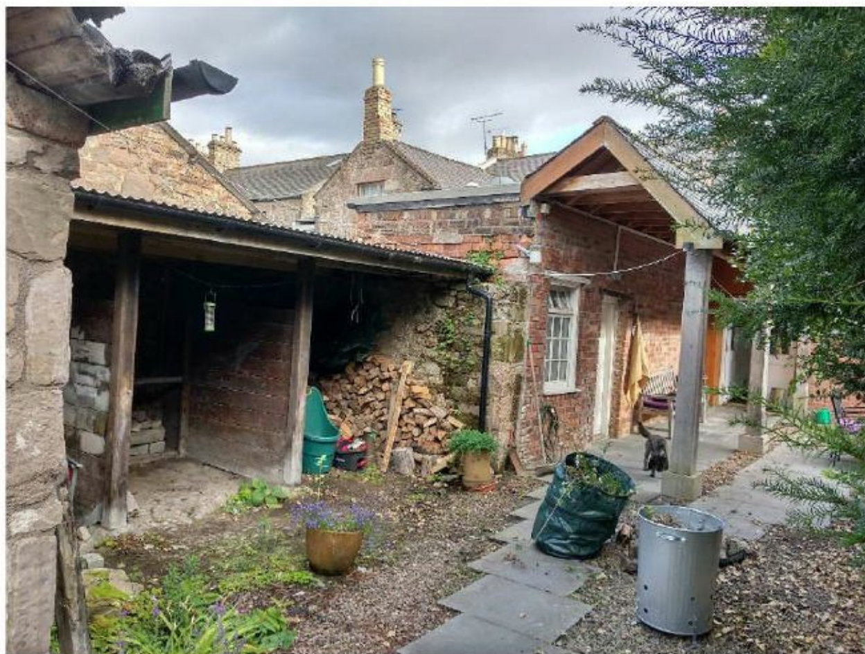
The Old Stable has three stone walls and can be retained, albeit beneath a new roof. The new roof will be made by extending the walkway/shower-room roof.
