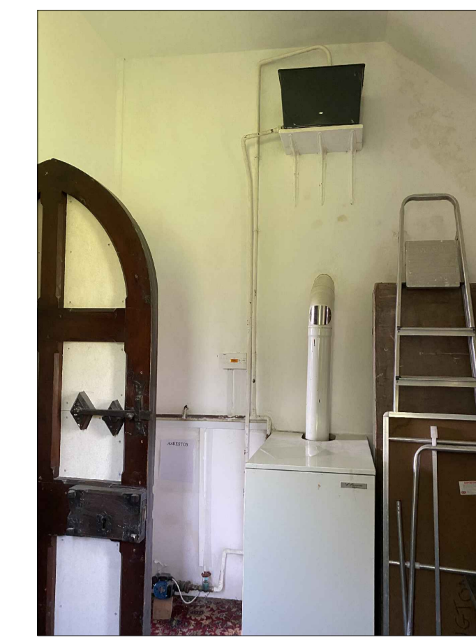
Existing boiler, flue and top up tank
