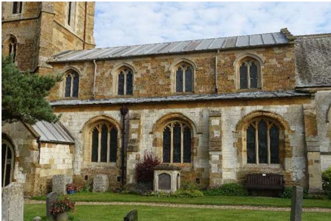
Figure 2: South Aisle roof slope largely hidden from view at ground level.
