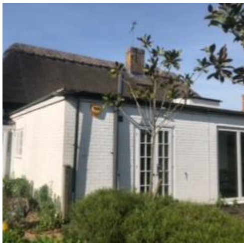
Back & side (roof damage clearly seen on corner)
