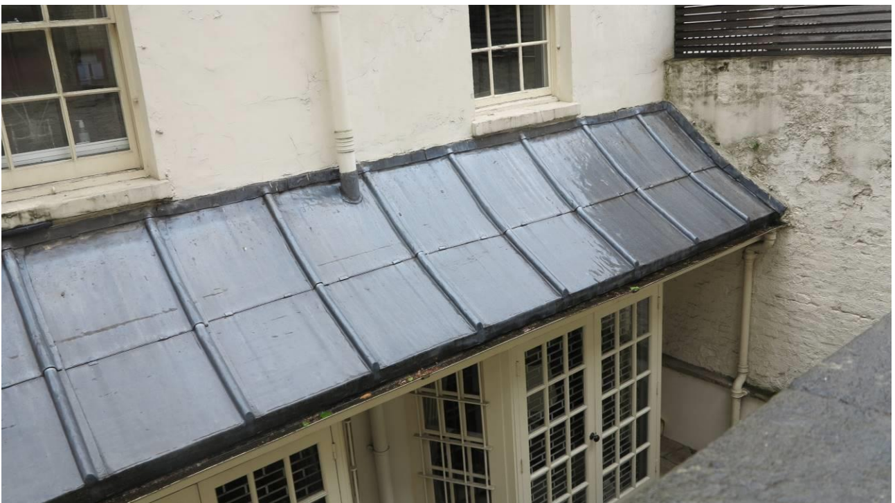
Plate 6. Looking down over the boundary wall separating the grounds of St. Peter's Church, Eaton Square from No.16 to the late 20 th -century additions to the rear elevation of No.16
