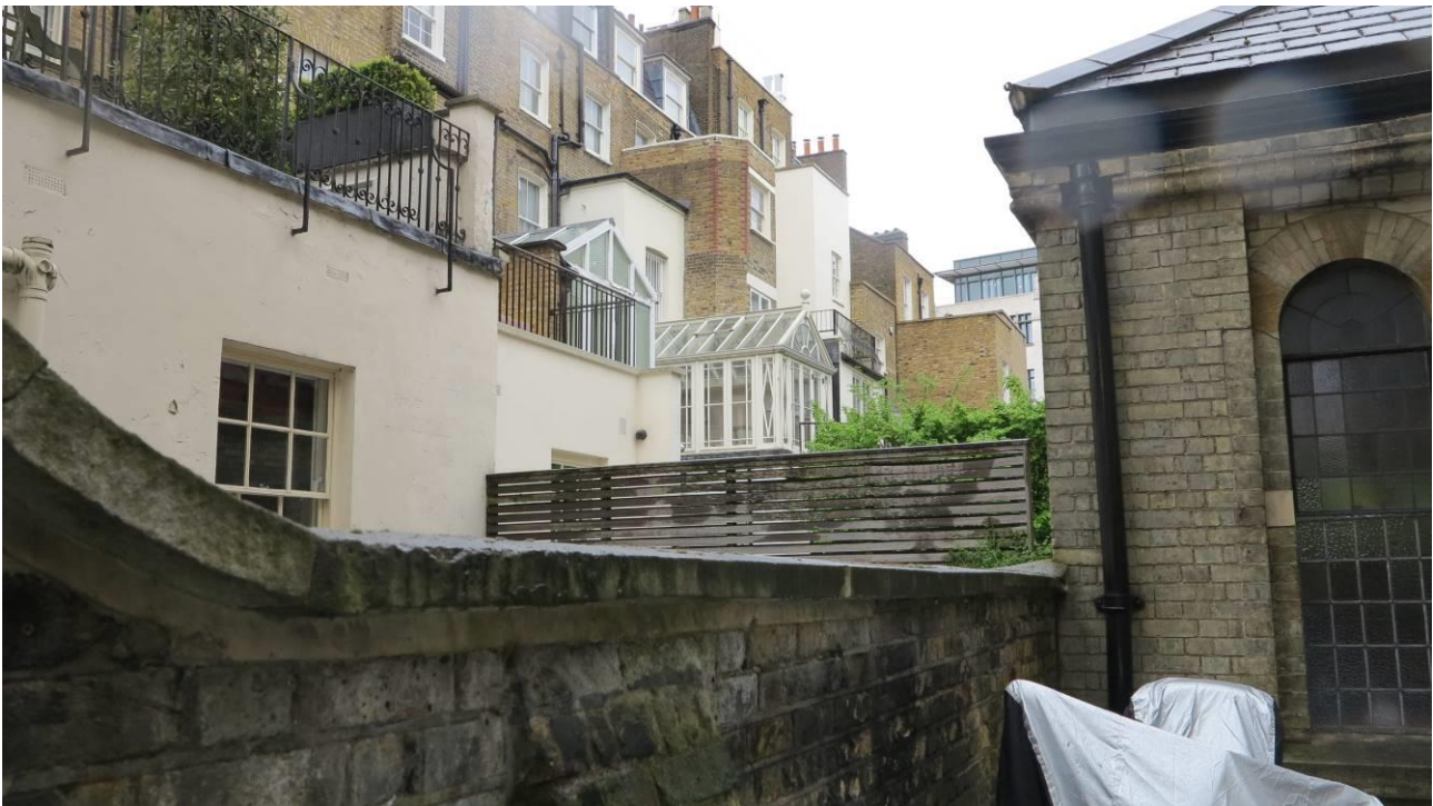
Plate 16. Late 20 th -century conservatory-like extensions sit on top of earlier flat-roofed extensions to the rear elevations of Nos.17 & 18
