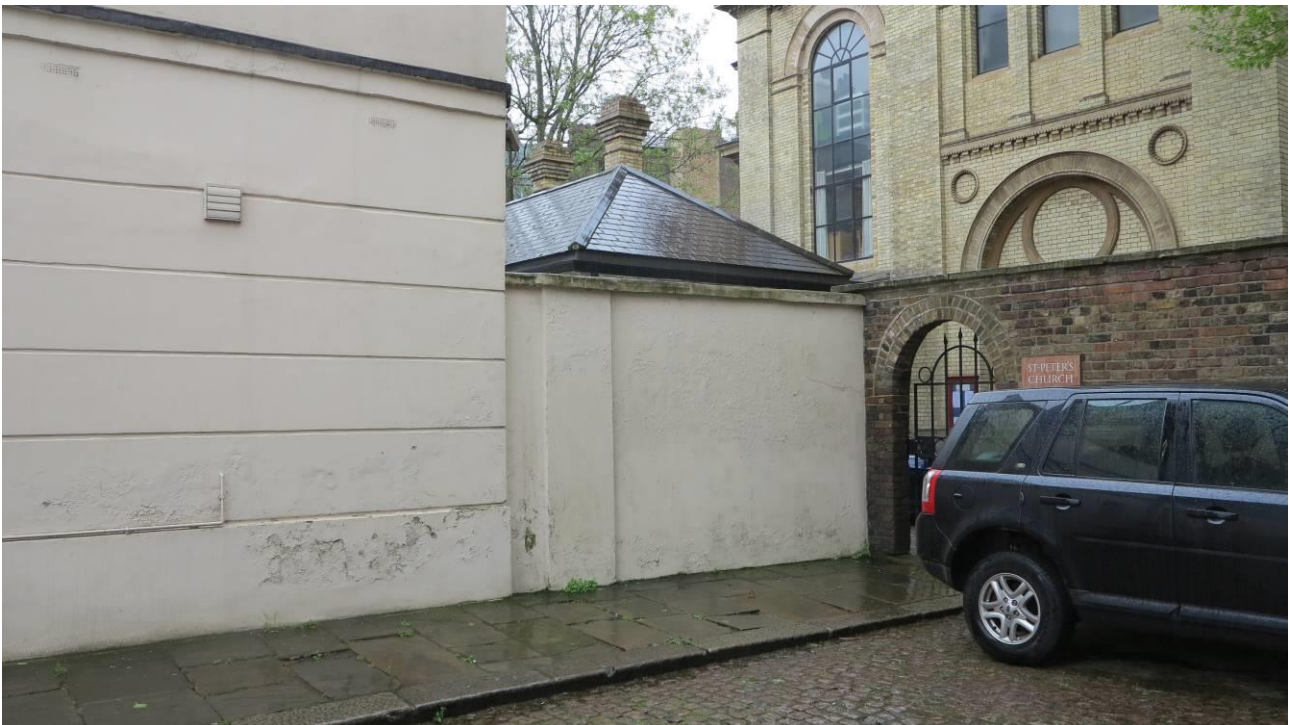
Plate 8. The flank (Wilton Mews) elevation to the rear extension to No.16 and the boundary wall to its rear yard area
