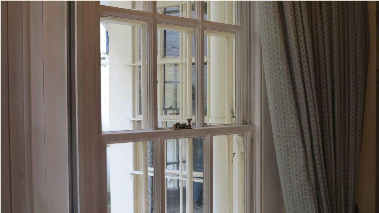
Plate 39. The 'horns' to the sash windows in the projecting bays to the living room and guest bedroom demonstrate that the bays date to the later 20 th century
