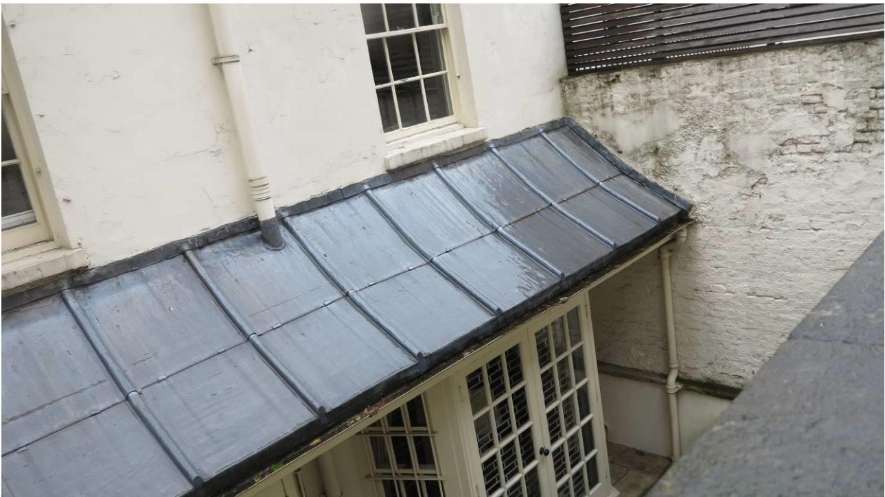
Plate 4. Looking down over the boundary wall separating the grounds of St. Peter's Church, Eaton Square from No.16 to the late 20 th -century additions to the rear elevation of No.16
