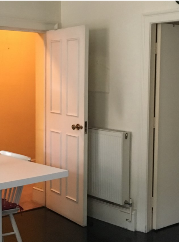
1 View of modern Kitchen door and door to maid's room showing modern planted panel beads and modern flush door leaf
